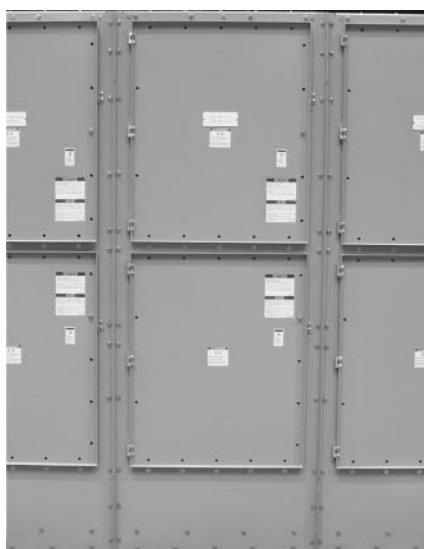
Rear View 5/15 kV VCP-W Arc-Resistant Switchgear
