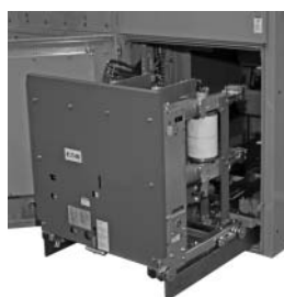
Breaker Shown Fully Withdrawn on Extension Rails
