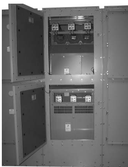
Rear View—Breaker Over Breaker Cable Termination
