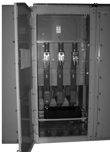
Rear View—Typical 27 kV Breaker Cable Termination
