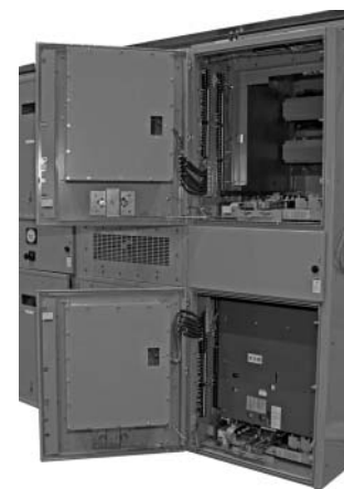
5/15 kV Breaker Over Breaker
