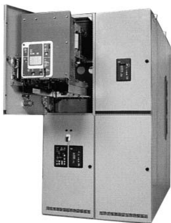
Fully Withdrawn Breaker
