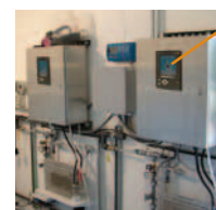
Field remote terminal.
