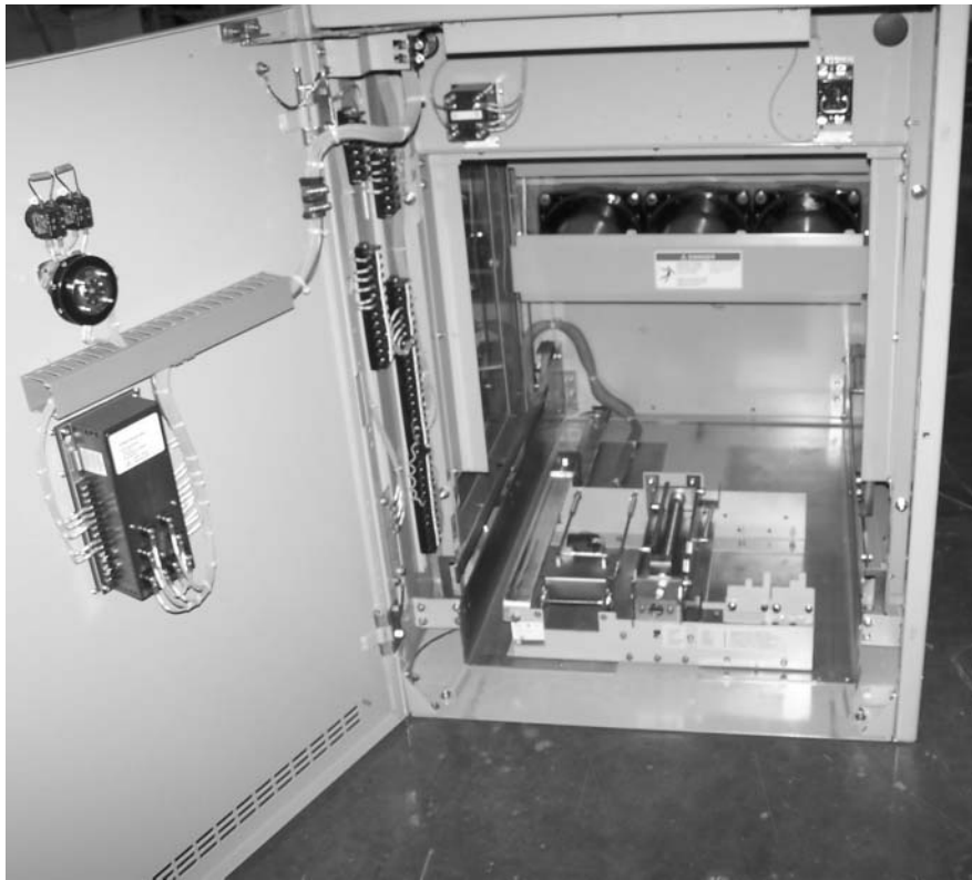
Roll-on-the-Floor Switchgear Compartment
