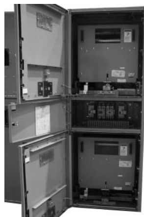
5/15 kV Auxiliary Over Auxiliary
