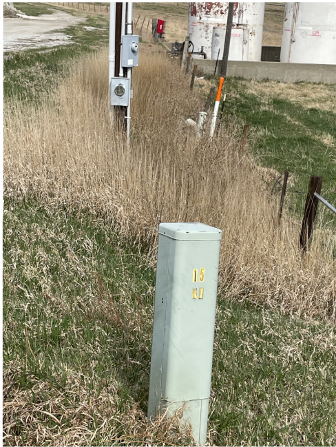
Conduit to building pedestal
