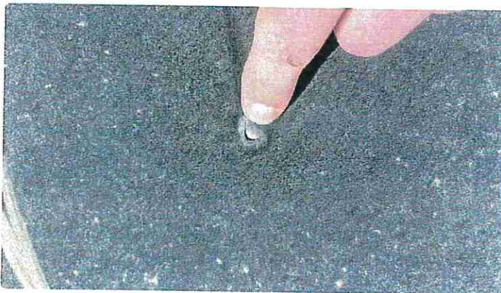
Photo showing an additional hole in the field membrane.
