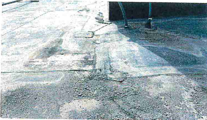
Photo showing area where water is ponding causing the membrane and base projection flashings to deteriorate.
