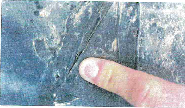
Photo showing water being pushed out of the inside corner wall flashings.
