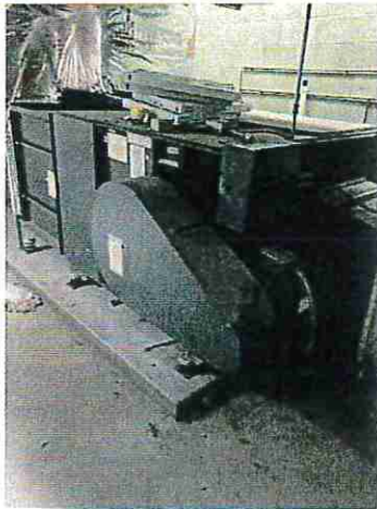
Air Handling Unit #3
