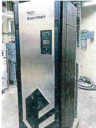
Middle School Boiler
