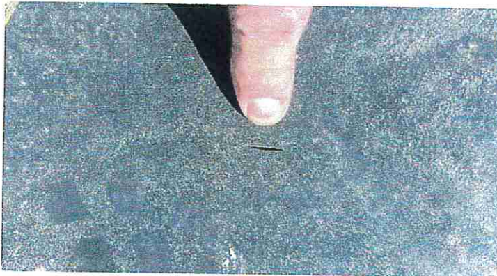
Photo showing an additional hole in the field membrane.
