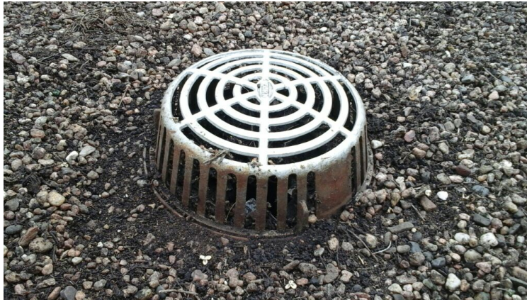
Photo showing drain cleared out.
