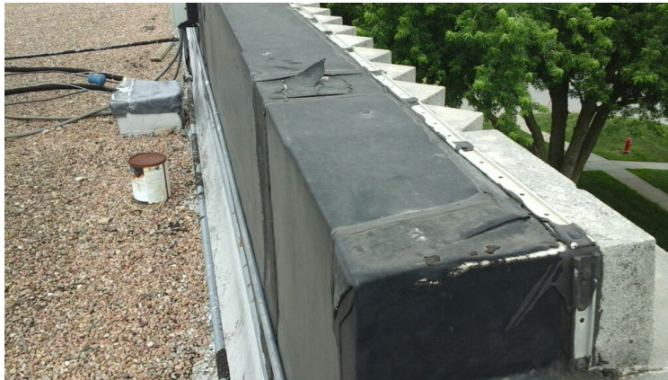
Photo showing rubber covering the concrete parapet wall deteriorating.
