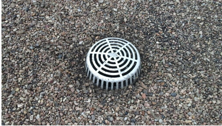
Photo showing condition of the drains.
