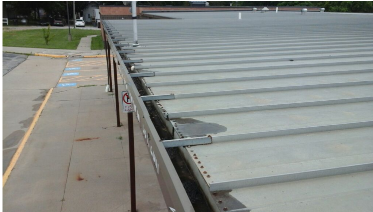
Photo showing condition of the gutter edge.
