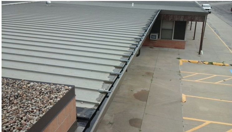
Photo showing clogged drain with full gutter.
