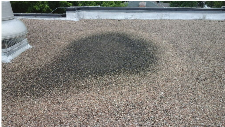
Photo showing evidence of ponding water.
