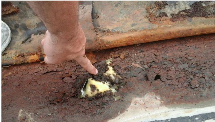
Photo showing a hole in the metal caused by rust under EPDM. This area is wide open and needs immediate attention.
