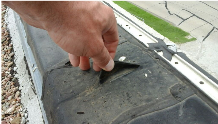
Photo showing torn patch covering seam in perimeter rubber. Concrete below is exposed to weather.
