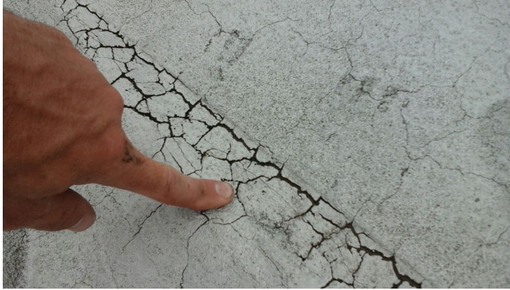
Photo showing a hole in the field membrane. Repaired as part of the maintenance agreement.
