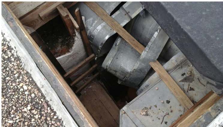
Photo showing dangerous access ladder next to crushed vent.
