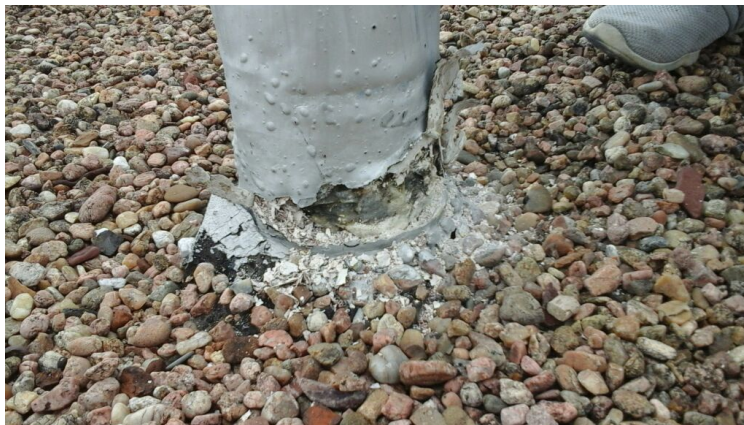
Photo showing lead pulling off and rusted around a vent projection. This is the most likely cause of the leak below. Repaired as part of the maintenance agreement.
