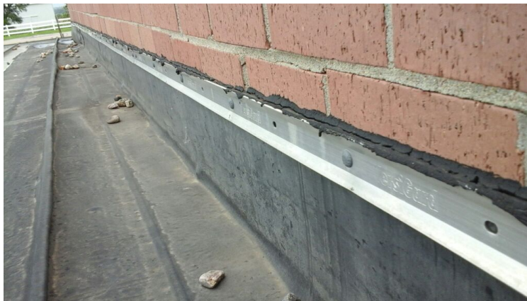
Photo showing ineffective term bar.
