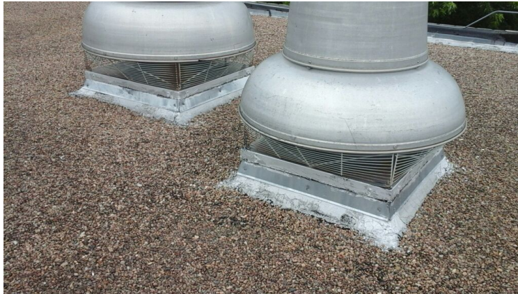
Photo showing condition of projection flashings.
