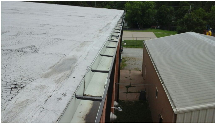
Photo showing condition of the gutter edge.
