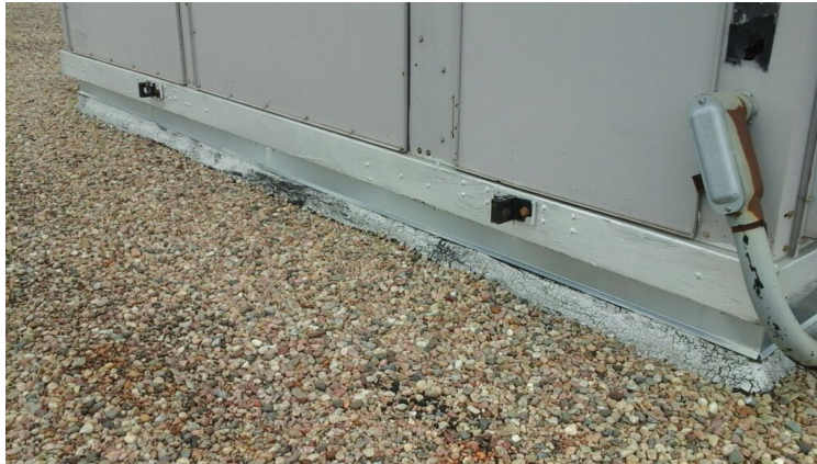
Photo showing condition of projection flashings. Minor alligatoring is occurring and should be monitored.
