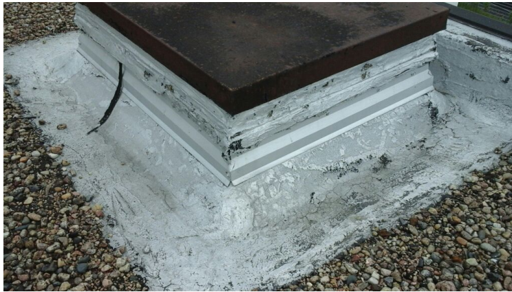
Photo showing condition of projection flashings.
