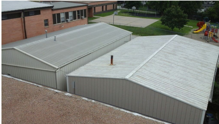
Photo showing additional overview of detached metal roofs.
