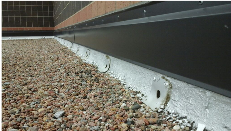
Photo showing condition of the perimeter flashings.
