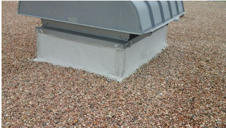
Photo showing condition of projection flashings.
