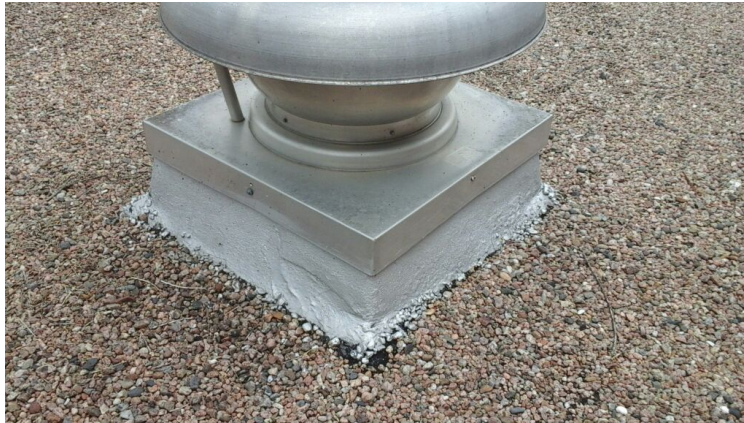
Photo showing condition of projection flashings.
