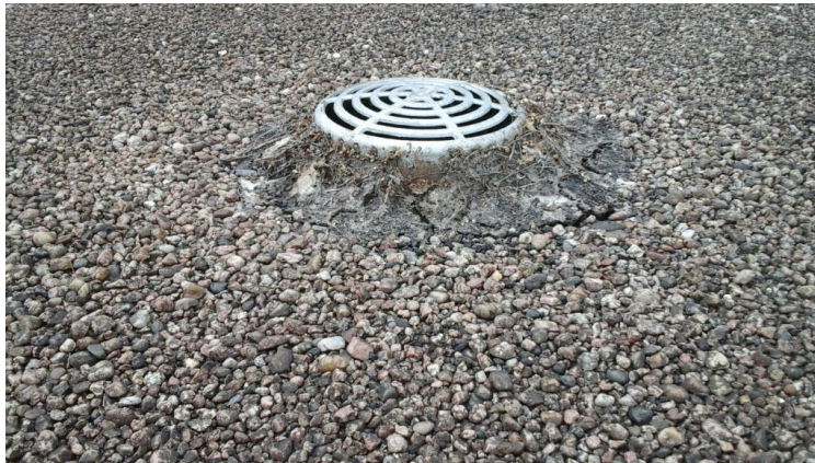
Photo showing clogged drain. Cleaned out as part of the maintenance agreement.
