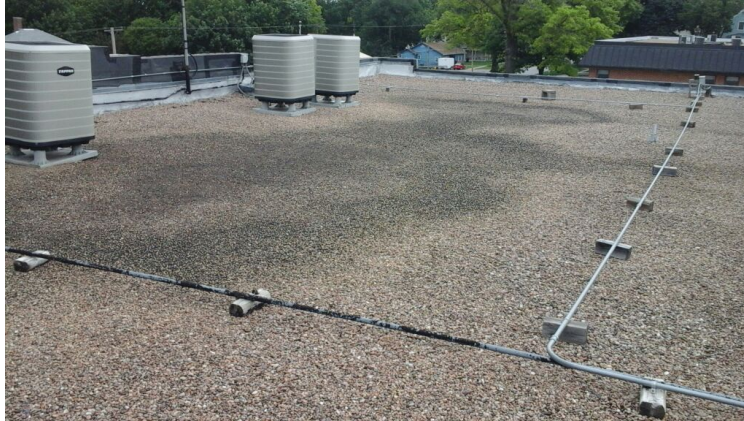
Photo showing evidence of ponding water.
