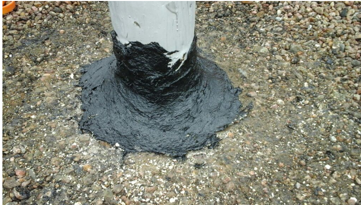
Photo showing repair made to the vent stack.
