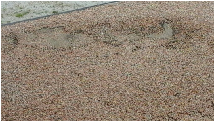
Photo showing deterioration of surfacing.
