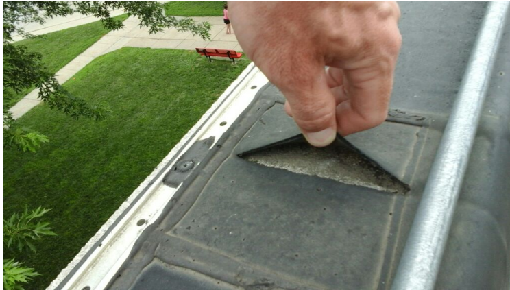
Photo showing a seam patch that is split and open to weather.
