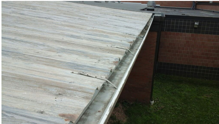
Photo showing condition of the gutter edge.
