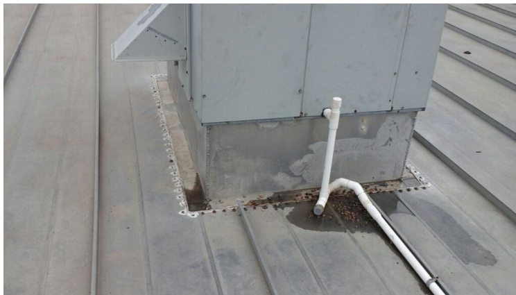
Photo showing condition of projection flashings.
