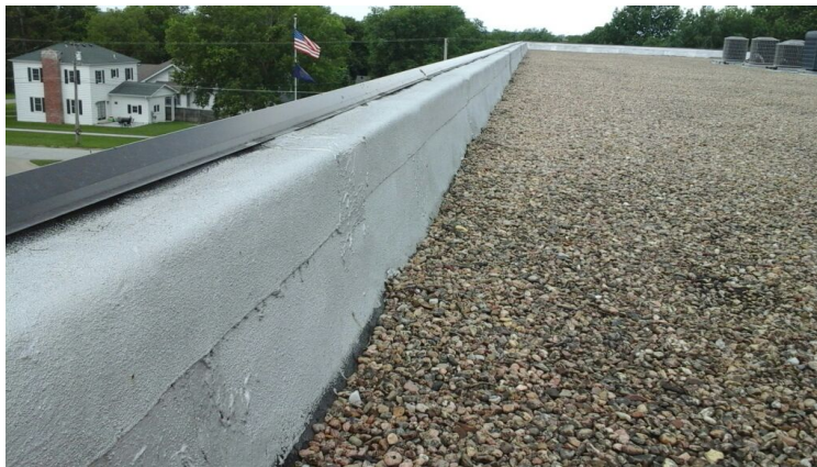
Photo showing condition of the perimeter flashings.
