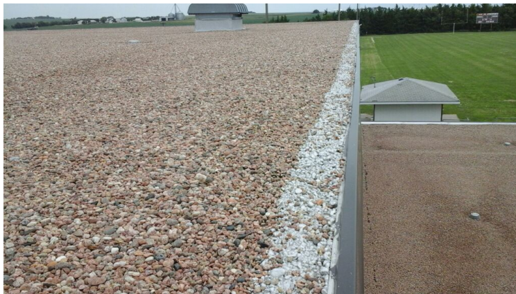
Photo showing condition of gravel stop metal.
