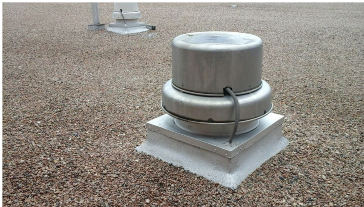
Photo showing condition of projection flashings.
