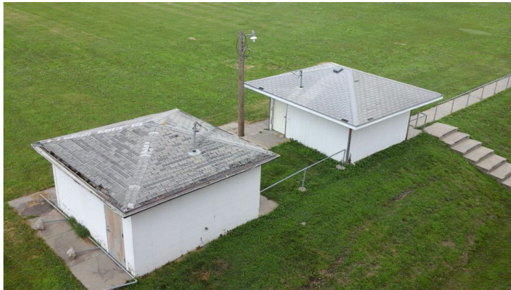
Photo showing condition of detached shingle roofs.
