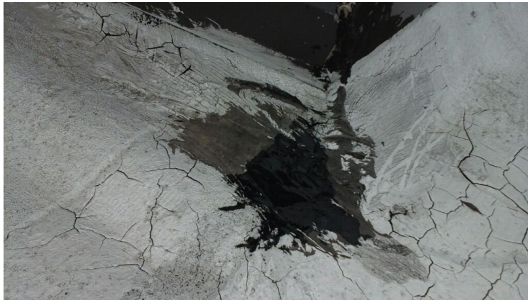
Photo showing a hole in he projection flashing. Patched as part of the maintenance agreement.
