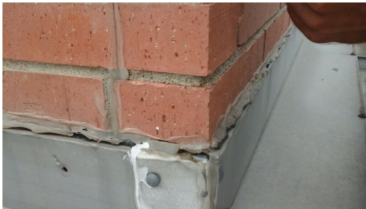
Photo showing silicone on top of caulking.
