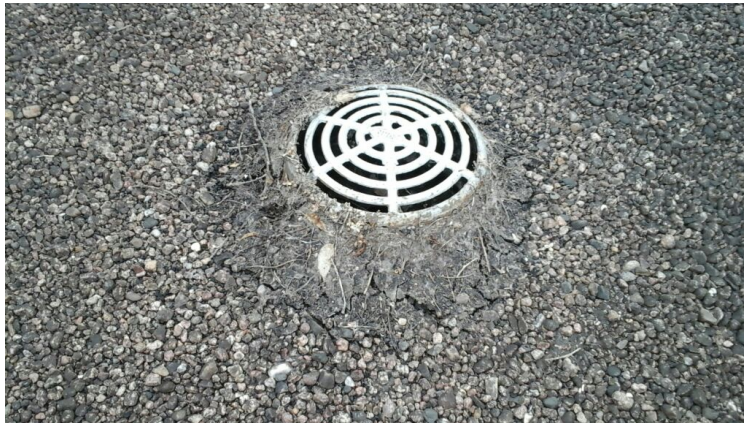
Photo showing clogged drain causing ponding water. Cleared out as part of the maintenance agreement.
