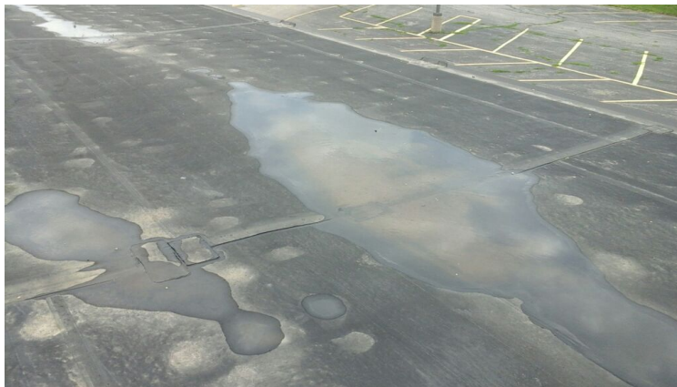
Photo showing ponding water.
