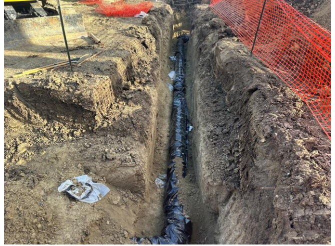
4/8: 12-inch suction line, photo looking north to Hickman Road.
