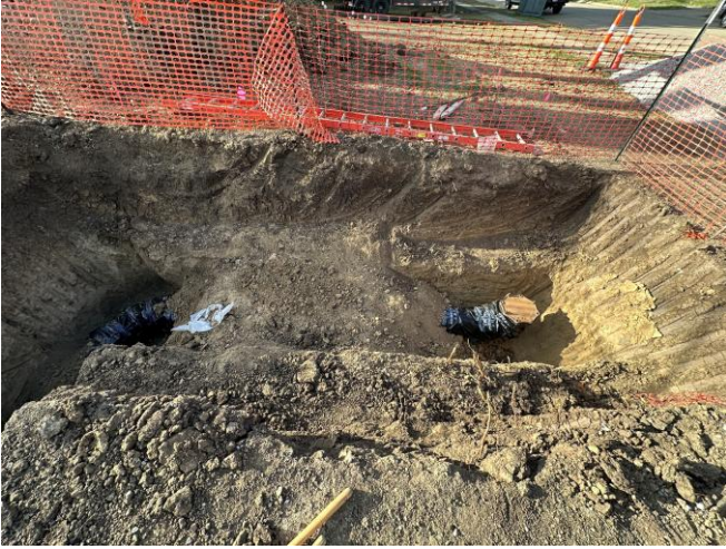
4/8: 12-inch suction line, connection for booster pump station.
