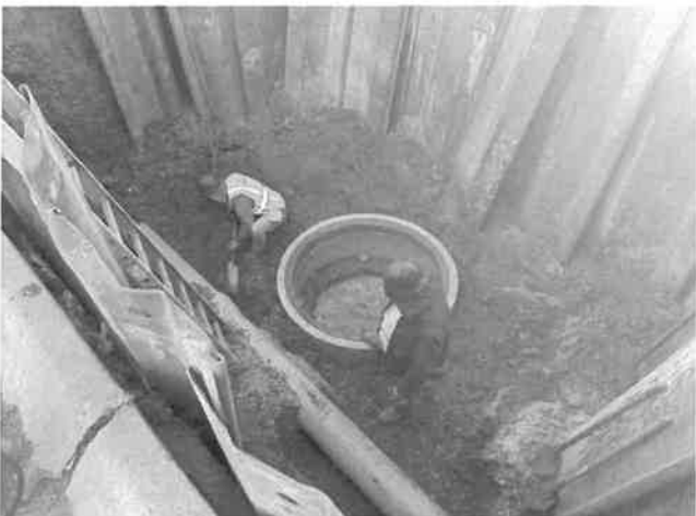
3/27: Installation of manhole base at Autumn Parkway. Prep for connection to existing water main.
