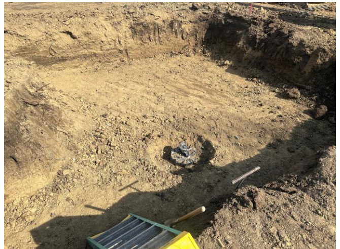
4/9: 12-inch suction line connection at booster pump station.
