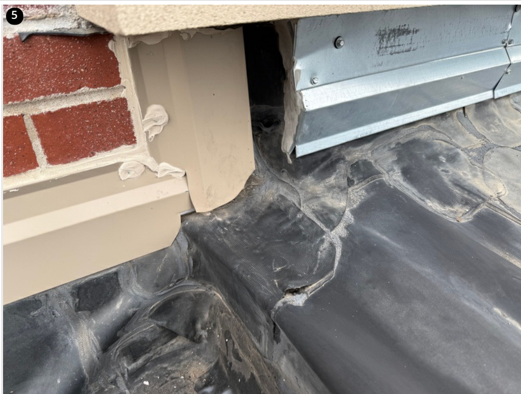
The corner and expansion detail has lead to multiple openings that have lead to leaks.
