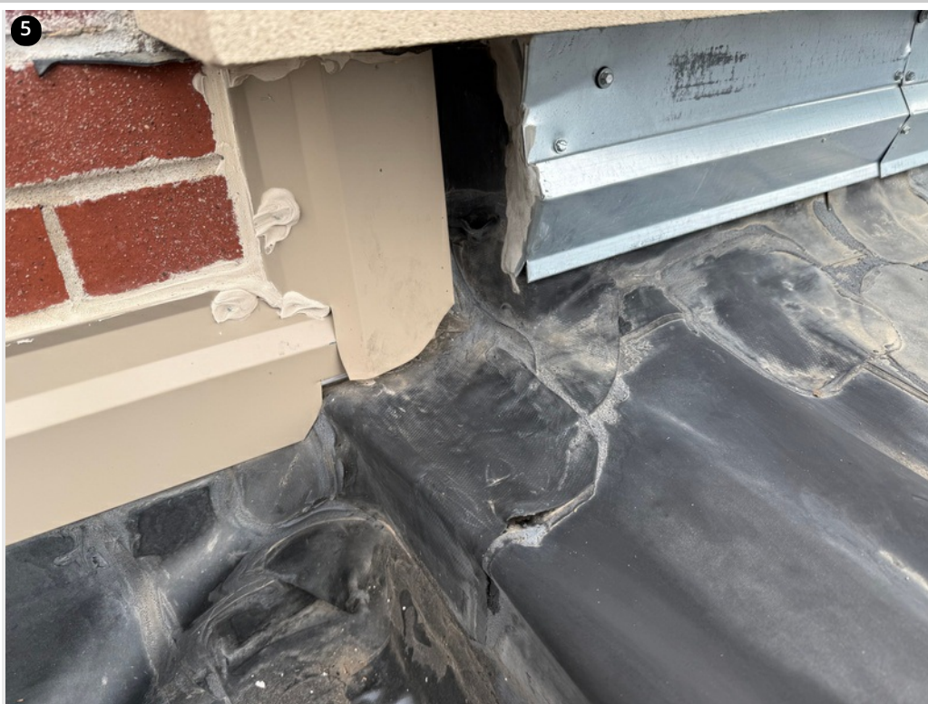
The corner and expansion detail has lead to multiple openings that have lead to leaks.
