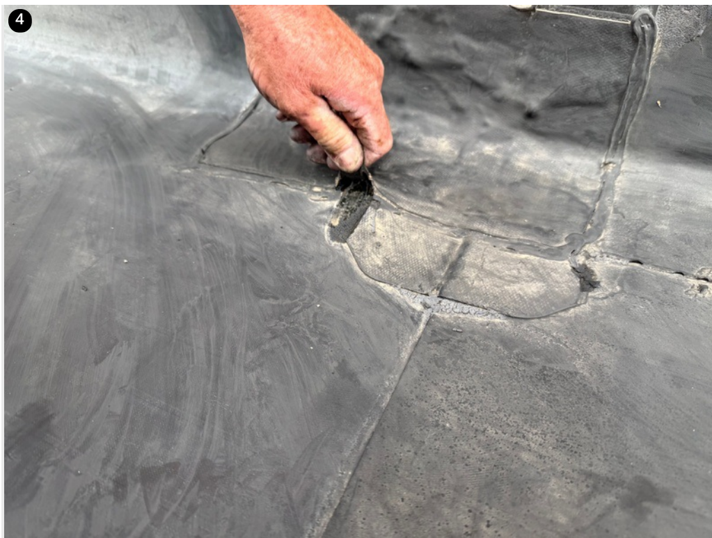
Each lap seam along the gym wall is showing signs of degradation. These matched with our 10 feet measurements.
