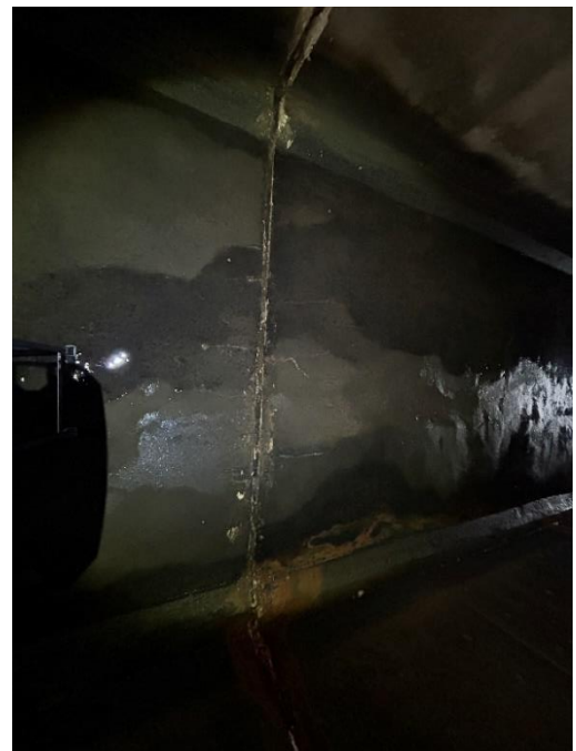
Location: Right Barrel – Joint C - Bottom Elevation Remarks: Joint filler in good condition. Joint Gap: 2” (typ.).
