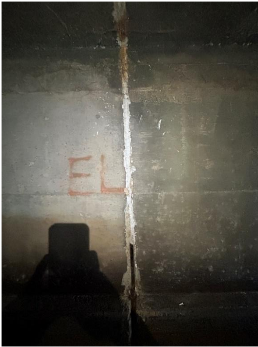
Location: Middle Barrel – Joint E - Left Elevation Remarks: Joint sealant (caulk) is missing from 0” to 24”. Oakum rope filler in poor condition. Joint sealant in poor condition from 42” to 48”. Joint Gap: 2.5” (typ.)
