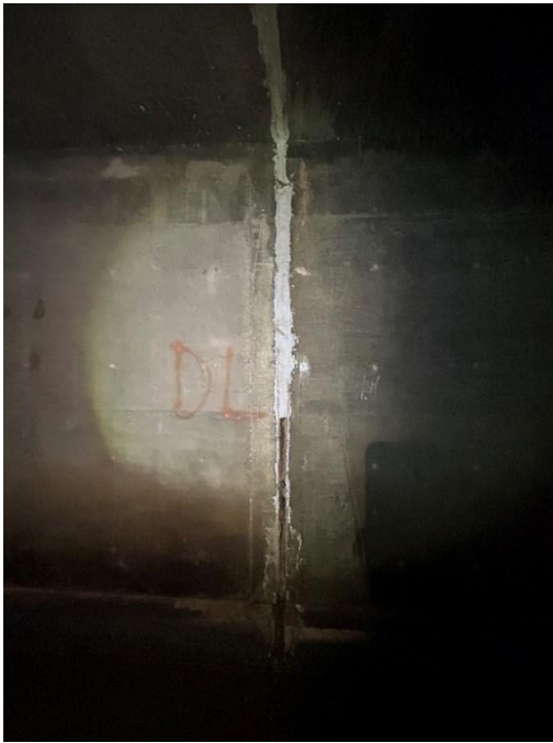
Location: Middle Barrel – Joint D - Left Elevation Remarks: Joint sealant (caulk) is missing from 0” to 47”. Oakum rope filler in poor condition. Joint Gap: 2.25” (typ.)
