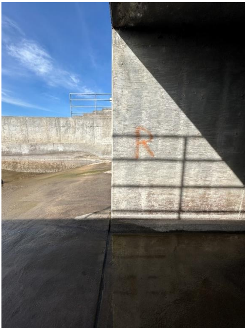
Location: Left Barrel – Joint F - Right Elevation
