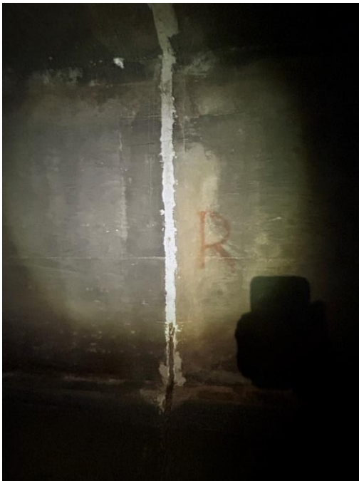
Location: Middle Barrel – Joint D - Right Elevation Remarks: Joint sealant (caulk) is missing from 0” to 24”. Oakum rope filler in moderate condition. Joint Gap: 1.75” (typ.)
