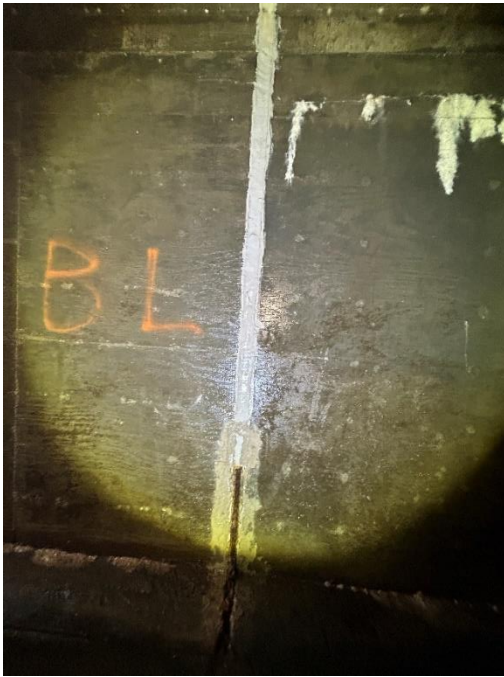
Location: Left Barrel – Joint B - Left Elevation Remarks: Joint sealant (caulk) is missing from 0” to 24”. Oakum rope filler in poor condition. Joint Gap: 2.5” (typ.)
