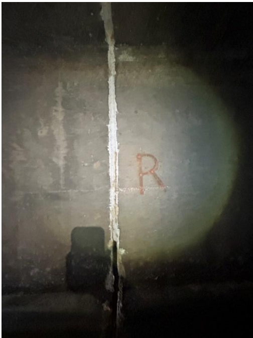
Location: Middle Barrel – Joint E - Right Elevation Remarks: Joint sealant (caulk) is missing from 0” to 28”. Oakum rope filler in poor condition. Joint Gap: 2.25” (typ.)
