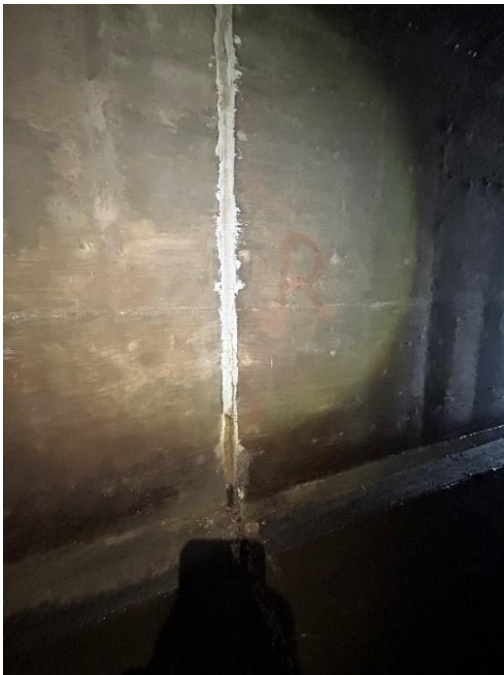
Location: Middle Barrel – Joint C - Right Elevation Remarks: Joint sealant (caulk) is missing from 0” to 24”. Oakum rope filler in poor condition. Joint sealant in poor condition from 24” to 42”. Joint Gap: 2.25” (typ.)
