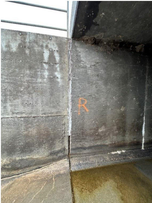
Location: Right Barrel – Joint F - Right Elevation Remarks: Joint sealant (caulk) is missing from 0” to 24”. Oakum rope filler in poor condition. Joint Gap: 2” (typ.)
