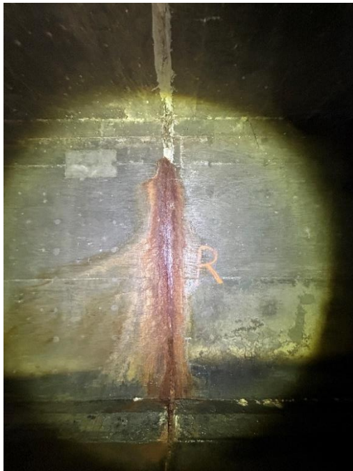
Location: Right Barrel – Joint D - Right Elevation Remarks: Joint sealant (caulk) is missing from 0” to 24”. Oakum rope filler in poor condition. Iron stain originates at joint a height of 98”. Joint Gap: 2” (typ.)
