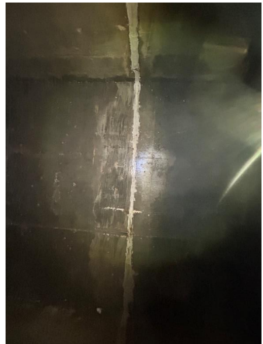
Location: Middle Barrel – Joint D - Top Elevation
