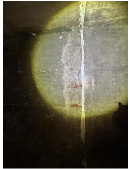
Location: Right Barrel – Joint D - Top Elevation Remarks: Minor cracking with iron stains.
