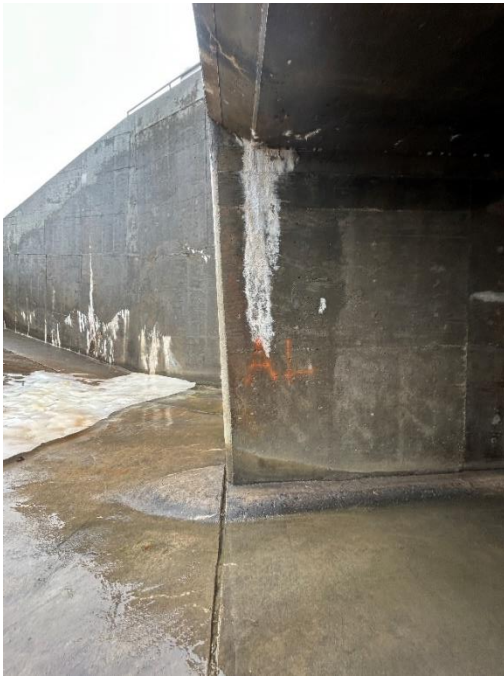
Location: Middle Barrel – Joint A - Left Elevation Remarks: Joint filler in good condition. Joint Gap: 1.5" (typ.)
