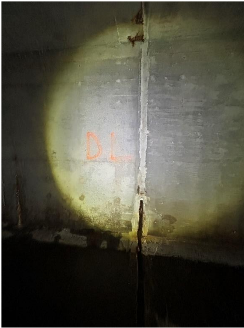
Location: Left Barrel – Joint D - Left Elevation Remarks: Joint sealant (caulk) is missing from 0” to 23”. Oakum rope filler in poor condition. Joint Gap: 3.25” (typ.)
