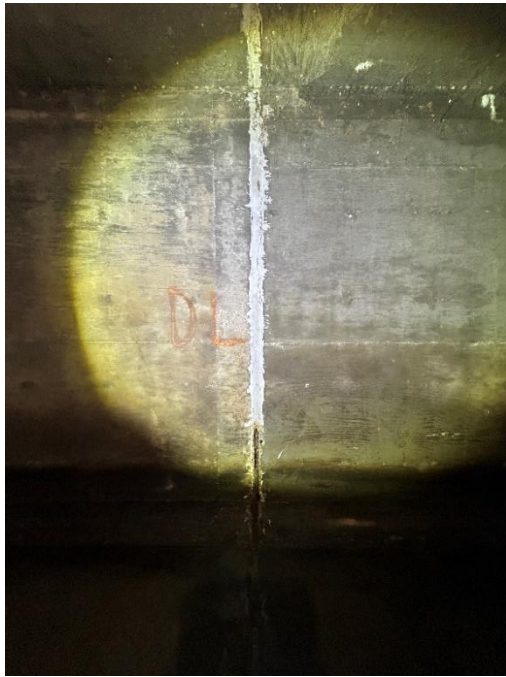
Location: Right Barrel – Joint D - Left Elevation Remarks: Joint sealant (caulk) is missing from 0” to 24”. Oakum rope filler in poor condition. Joint Gap: 2” (typ.)
