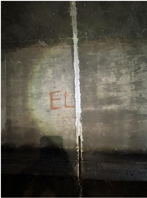
Location: Right Barrel – Joint E - Left Elevation Remarks: Joint sealant (caulk) is missing from 0” to 24”. Oakum rope filler in poor condition. Joint Gap: 2.5” (typ.)
