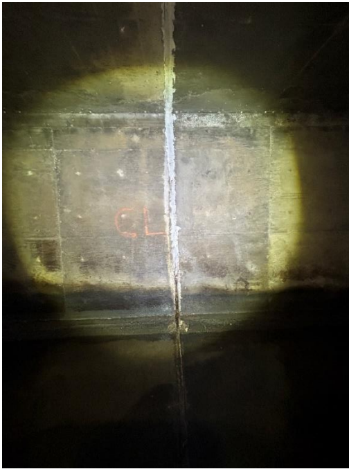
Location: Right Barrel – Joint C - Left Elevation Remarks: Joint sealant (caulk) is missing from 0” to 24”. Oakum rope filler in poor condition. Joint Gap: 3” (typ.)
