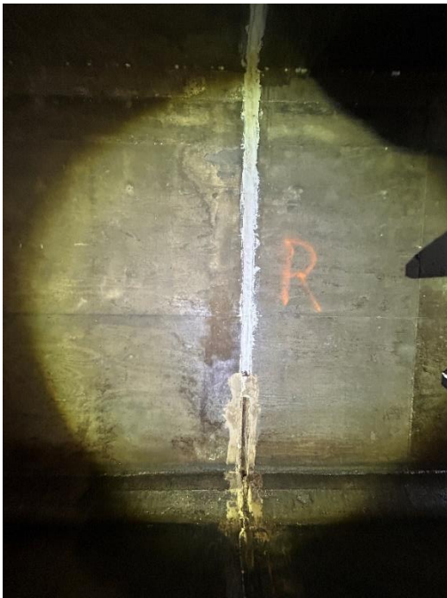
Location: Left Barrel – Joint B - Right Elevation Remarks: Joint sealant (caulk) is missing from 0” to 24”. Oakum rope filler in poor condition. Joint Gap: 3” (typ.)
