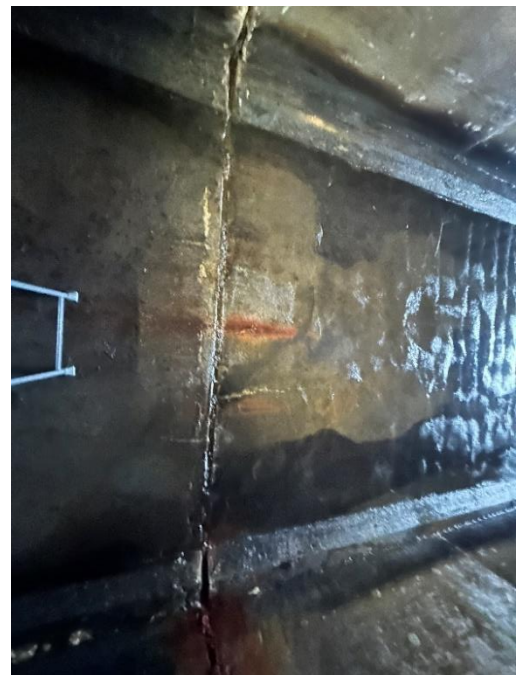
Location: Right Barrel – Joint D - Bottom Elevation Remarks: Joint filler in good condition along base, poor at chamfers. Joint Gap: 2” (typ.).
