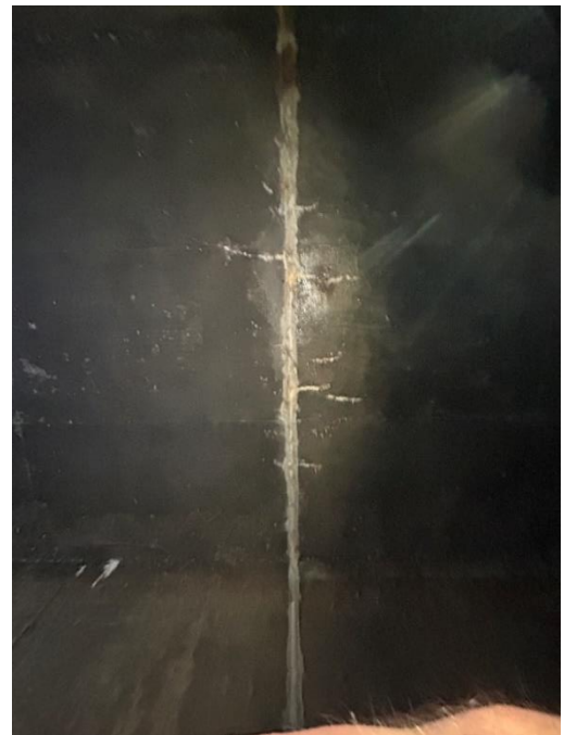
Location: Middle Barrel – Joint E - Top Elevation Remarks: Minor cracking with efflorescence.
