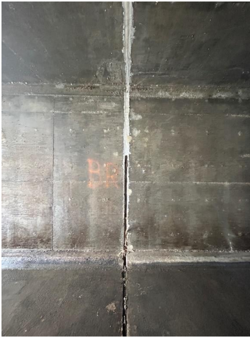
Location: Middle Barrel – Joint B - Left Elevation Remarks: Joint sealant (caulk) and filler is missing from 0” to 66”. Void extends into adjacent RCB. Joint Gap: 3” (typ.)
