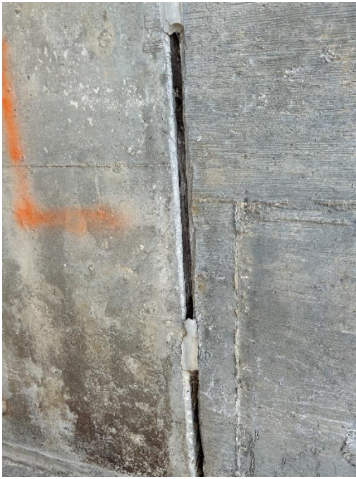
Location: Left Barrel – Joint F - Left Elevation Remarks: Joint filler in poor condition from 0” to 24.25”. Sealant missing or ineffective from 0” to 60.75”. Joint Gap: 1.75” (typ.)
