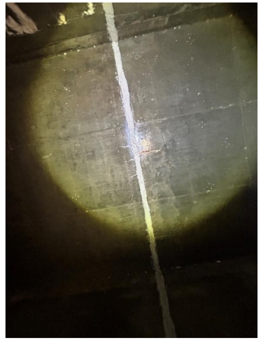
Location: Left Barrel – Joint B - Top Elevation Remarks: Minor crack with iron stain near midspan.
