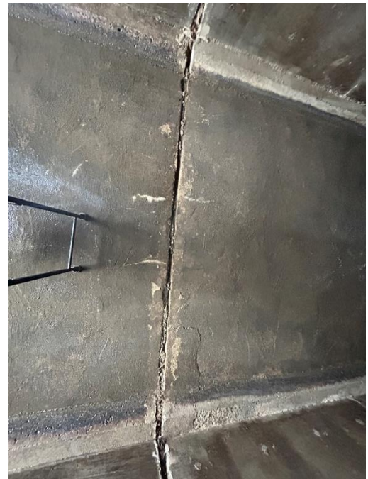
Location: Middle Barrel – Joint B - Bottom Elevation Remarks: Joint filler in moderate condition. Joint filler typically begins at depth of 1.5”, with peak at 3”. Joint Gap: 1.5” (typ.)
