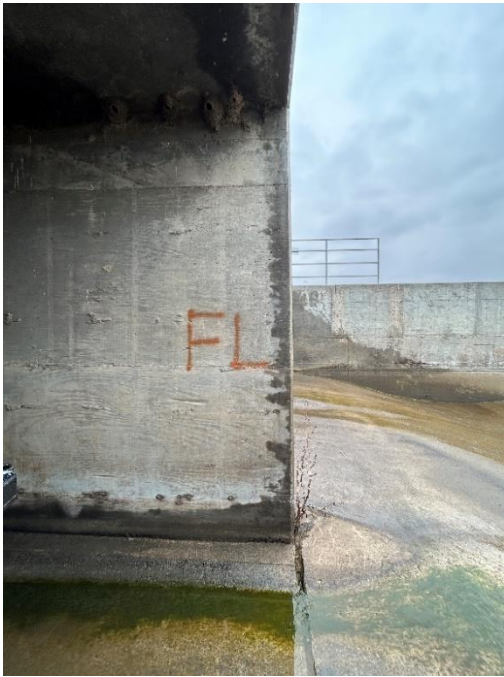
Location: Right Barrel – Joint F - Left Elevation Remarks: Longitudinal spalling projects upstream 12” at the chamfer to wall transition.
