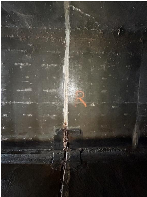
Location: Right Barrel – Joint E - Right Elevation Remarks: Joint sealant (caulk) is missing from 0” to 24” and in poor condition from 24” to 28”. Oakum rope filler in poor condition from 0” to 24”. Joint Gap: 2.25” (typ.)
