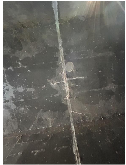
Location: Right Barrel – Joint E - Top Elevation Remarks: Minor cracking efflorescence.
