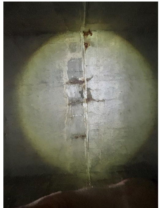
Location: Left Barrel – Joint D - Top Elevation Remarks: Minor cracking with iron stains.
