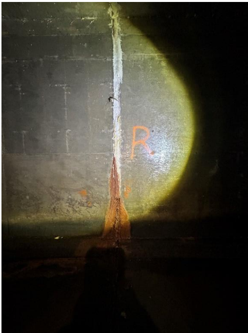
Location: Right Barrel – Joint C - Right Elevation Remarks: Joint sealant (caulk) is missing from 0” to 24”. Oakum rope filler in poor condition. Iron stain originates at joint a height of 48”. Joint Gap: 3” (typ.)
