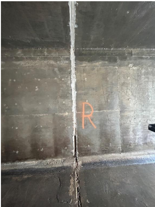
Location: Middle Barrel – Joint B - Right Elevation Remarks: Joint sealant (caulk) is missing from 0” to 24”. Oakum rope filler in poor condition. Joint Gap: 2.75” (typ.)
