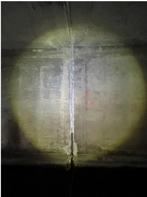
Location: Left Barrel – Joint D - Right Elevation Remarks: Joint sealant (caulk) is missing from 0” to 24.5”. Oakum rope filler in moderate condition. Joint Gap: 2.75” (typ.)
