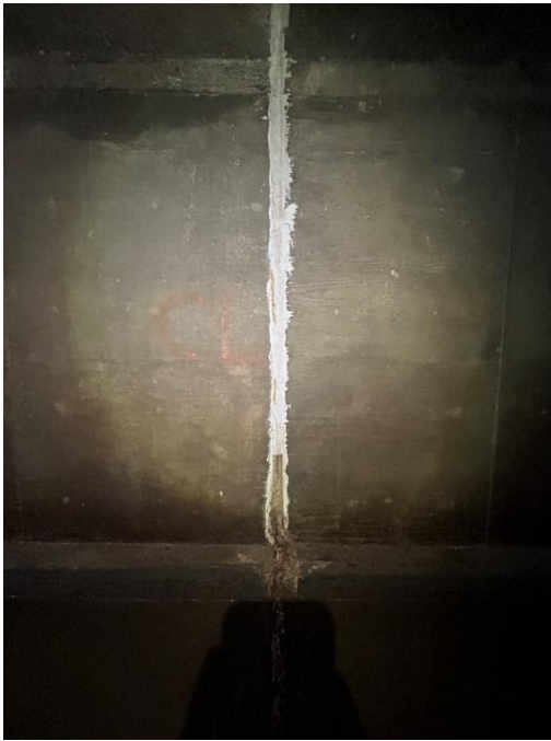
Location: Middle Barrel – Joint C - Left Elevation Remarks: Joint sealant (caulk) is missing from 0” to 24.5”. Oakum rope filler in poor condition. Joint Gap: 3” (typ.)
