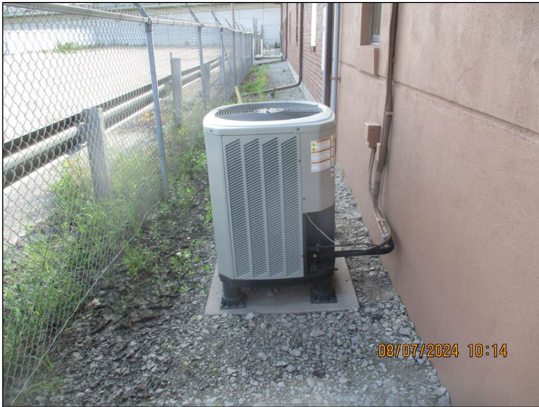
31001 Building- Central Air
