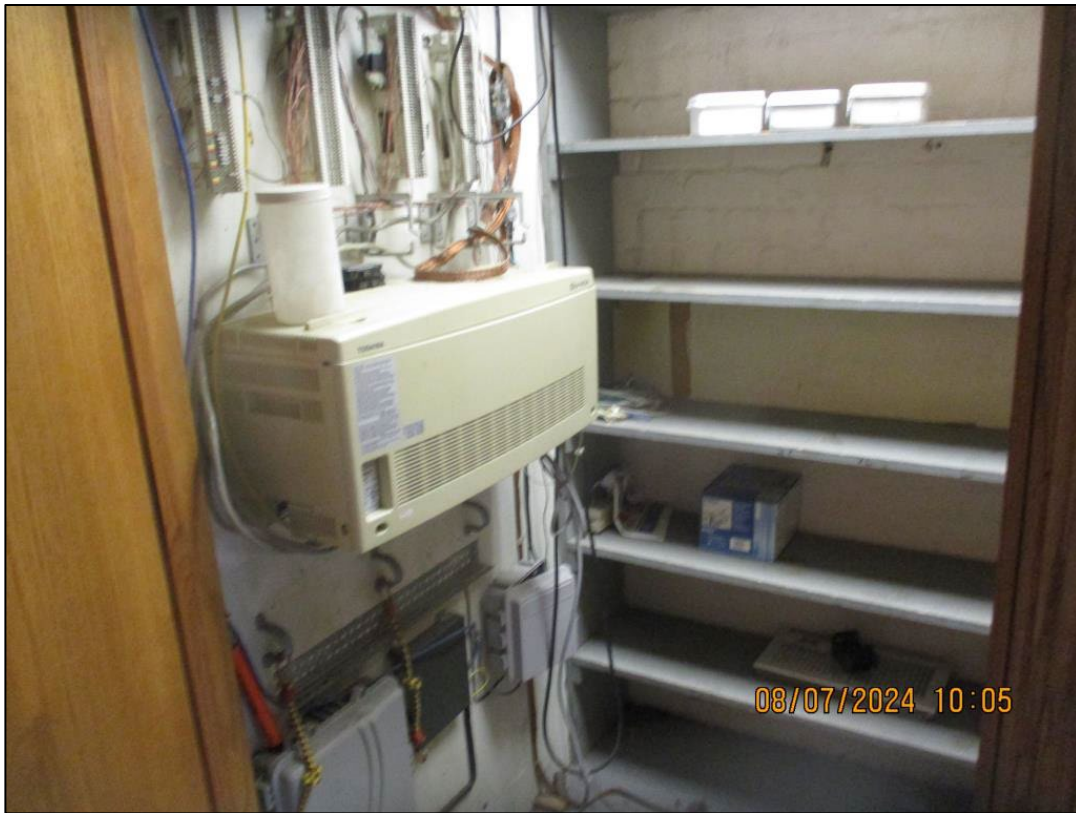
31001 Building- Electrical Room
