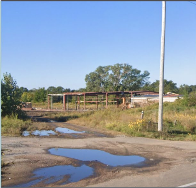
Post Flood Condition
