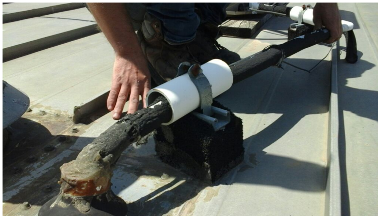
Photo showing insulation and silicone used to improperly penetrate roof. Could eventually cause leaks as it deteriorates
