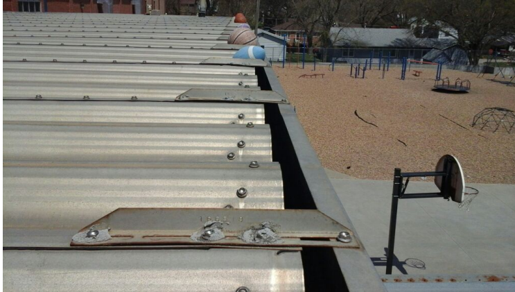
Photo showing condition of the gutter edge.
