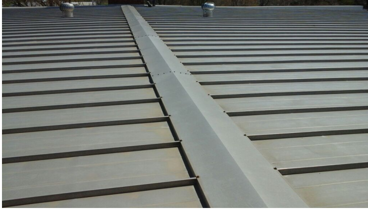
Photo showing condition of the ridge cap.
