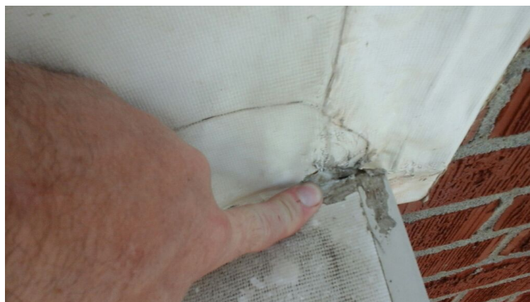
Photo showing hole in corner flashing that was sealed with silicone.
