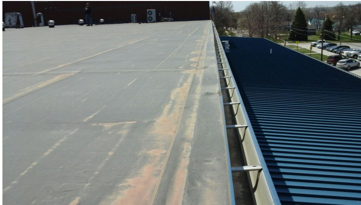
Photo showing condition of gutter edge.
