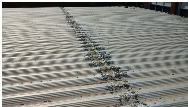
Additional photo of deteriorating seam coating.
