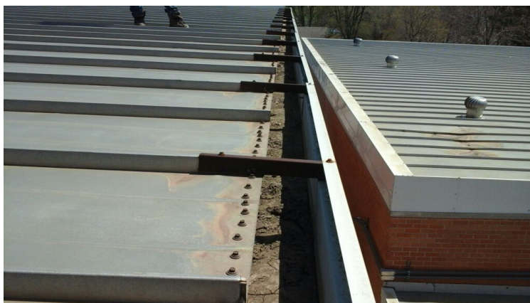
Photo showing condition of the gutter edge.
