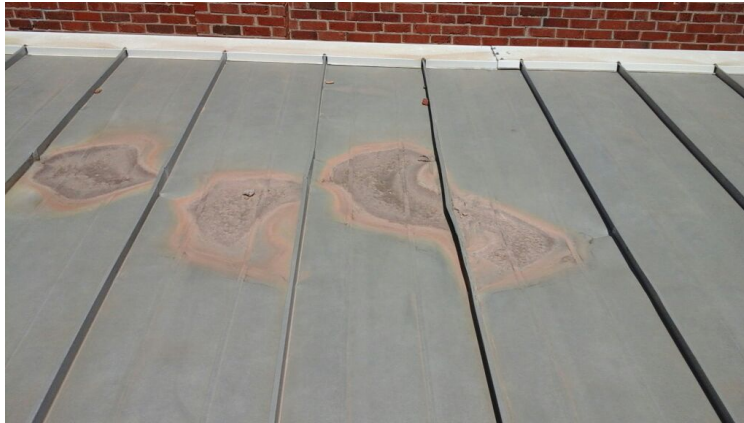
Photo showing damage to metal and standing seam where ponding water occurs.
