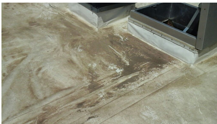
Photo showing evidence of ponding water.
