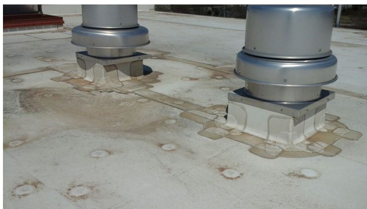
Photo showing condition of the projection flashings.
