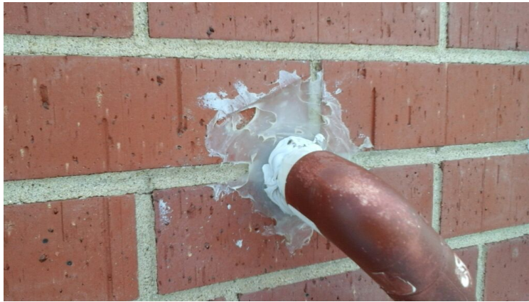
Photo showing projection in wall caulked with silicone.
