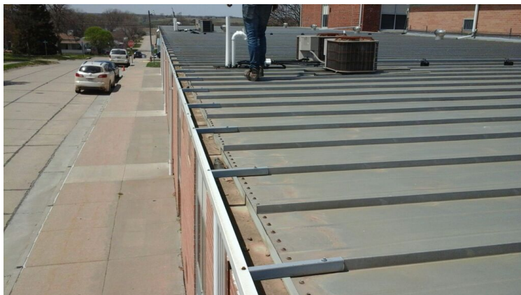
Photo showing condition of the gutter edge.
