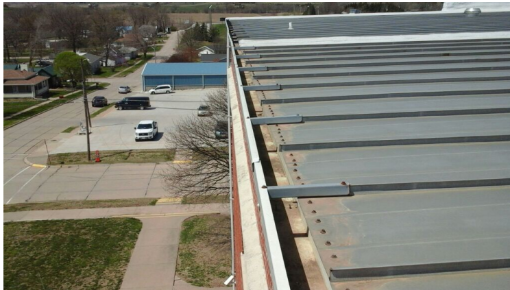
Photo showing condition of gutter edge.
