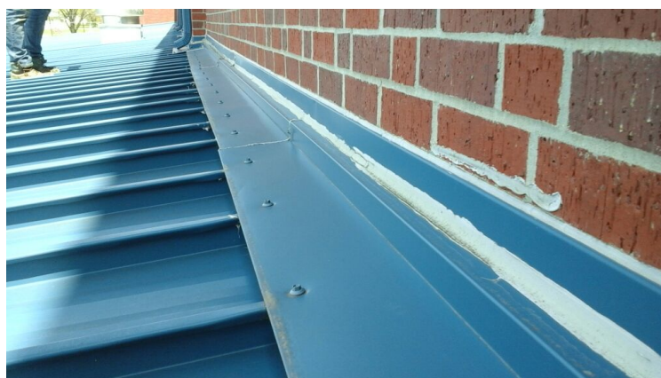
Photo showing condition of perimeter metal.
