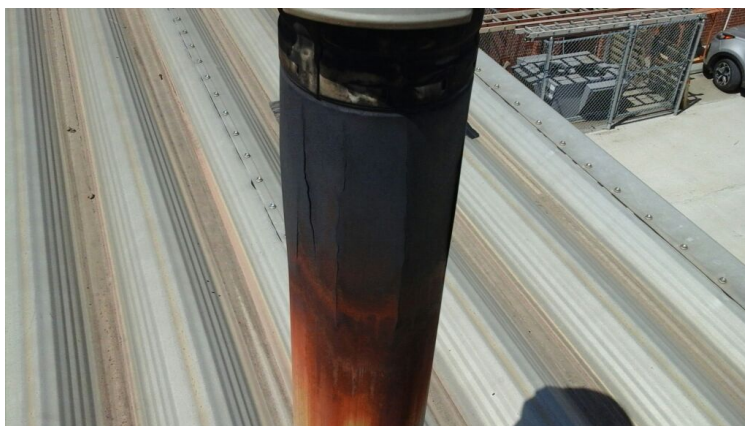
Photo showing cracked vent pipe.
