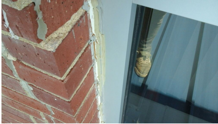
Photo showing caulk on top of caulk. Old layer must be removed before new layer can be applied.
