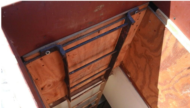
Photo showing hatch ladder with improper clearance for rungs at top.
