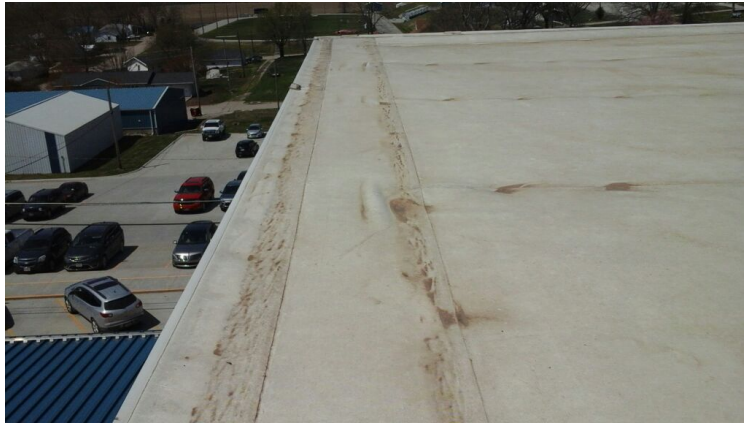
Photo showing condition of perimeter edge.
