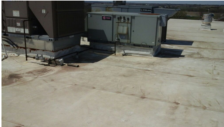
Photo showing HVAC units that have been replaced and need to be replaced.
