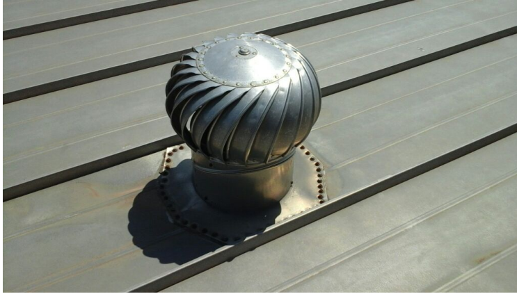
Photo showing condition of the penetrations.
