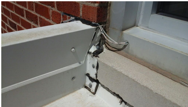
Photo showing corner with deteriorating caulking.
