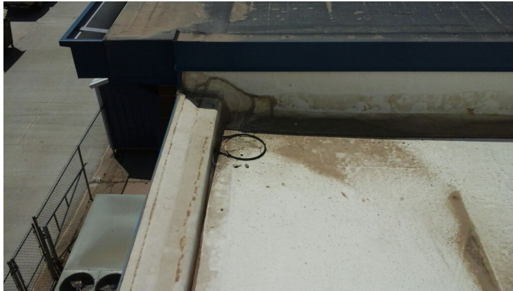
Photo showing condition of perimeter edge.
