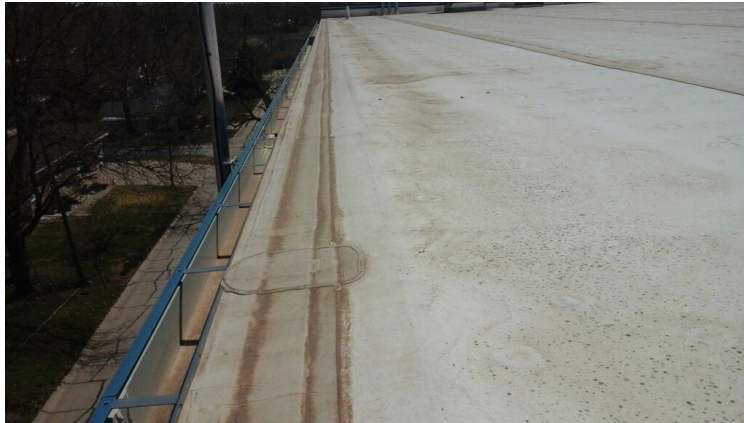
Photo showing condition of gutter edge.
