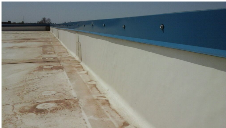
Photo showing condition of perimeter flashings.
