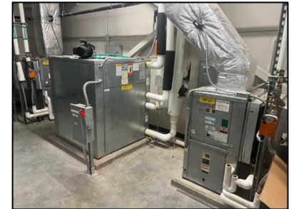
Penthouse Heat Pumps
