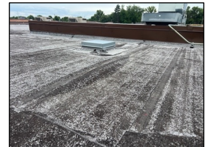
20+ Year Old Failing Roof
