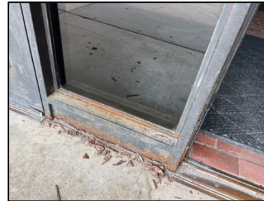
Rusted Single Pane Window
