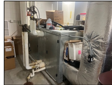
Typical Exposed Heat Pump
