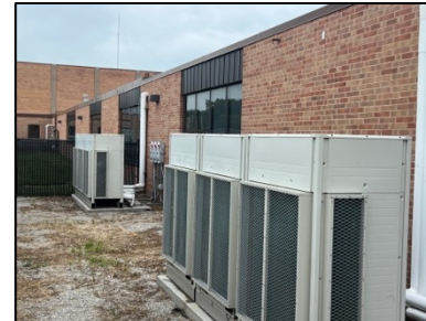
Outdoor VRF Units
