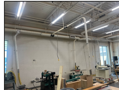
Existing Shop Exhaust System
