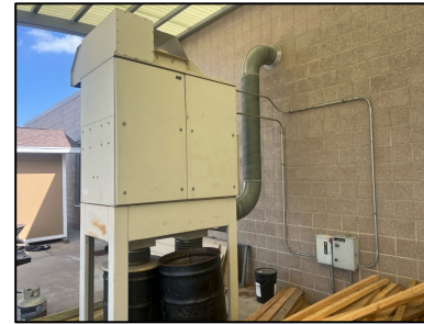
Outdoor Exhaust for Shops
