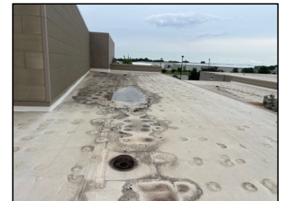
Slight Ponding on Roof
