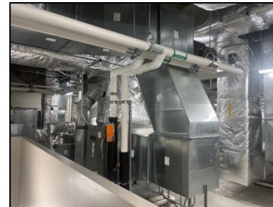
Penthouse Heat Pumps
