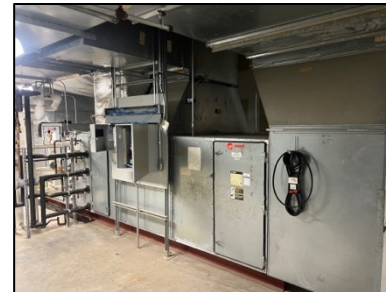
Penthouse Air Handler
