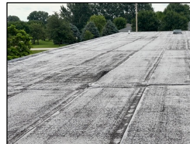
Buckling/Bubbled Rubber Roof
