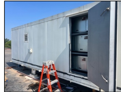
Heat Pumps in Penthouse
