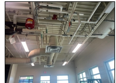
Exposed Weight Room Heat Pump
