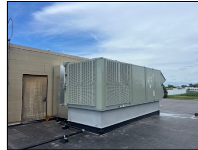
2025 Trane 40-ton Unit
