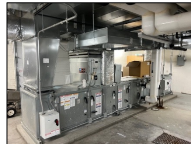
Daikin Air Handlers Installed 2017
