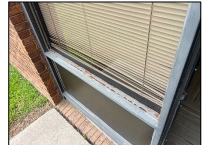
Rusted Single Pane Window
