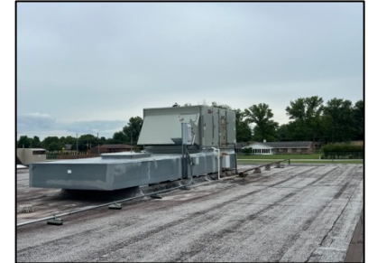
Trane Packaged Rooftop Unit
