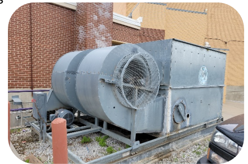
High School Cooling Tower – circa 1995
