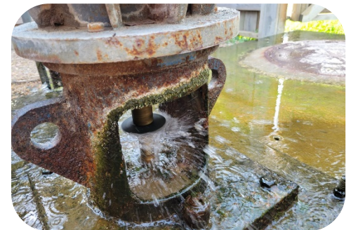
Middle School – Cooling Tower Pumps
