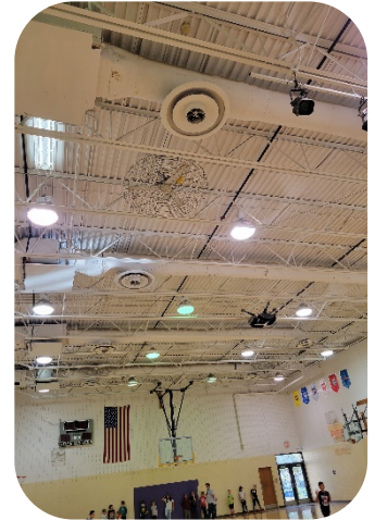
Hayward Elementary Gym – Water Source Heat Pumps
