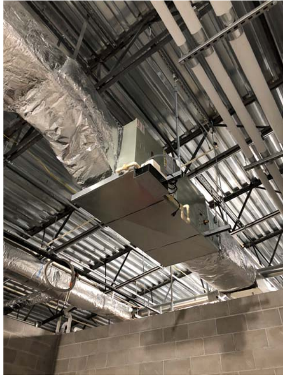
Furnace in Girl's Locker Room
