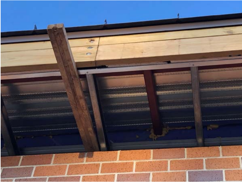
Splice in sub fascia missing bolts
