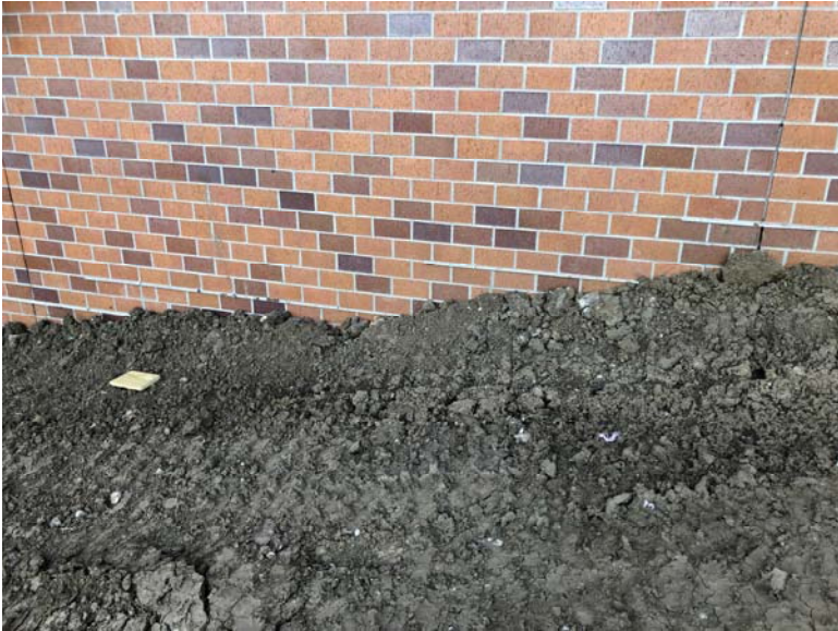
Backfill should not cover weeps in brick
