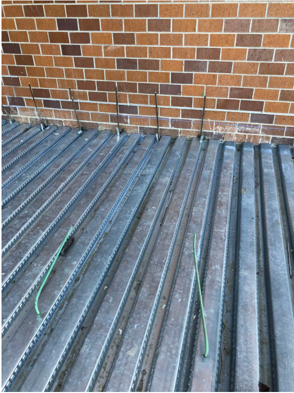
East ramp standard bar at wall should be epoxy coated
