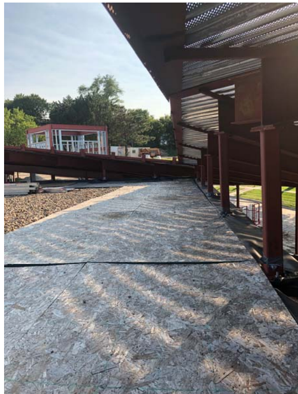
On the roof of the existing middle school wing. Roof protection is in place.
