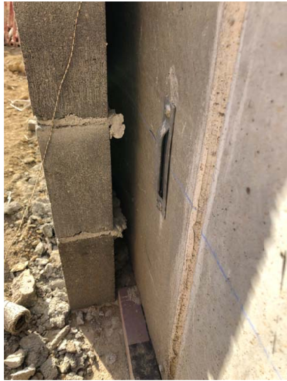
No grout behind block
