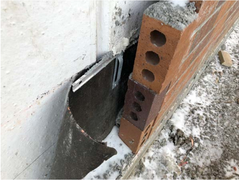
Base wall flashing (be sure to seal top of flashing at joints in precast wall)
