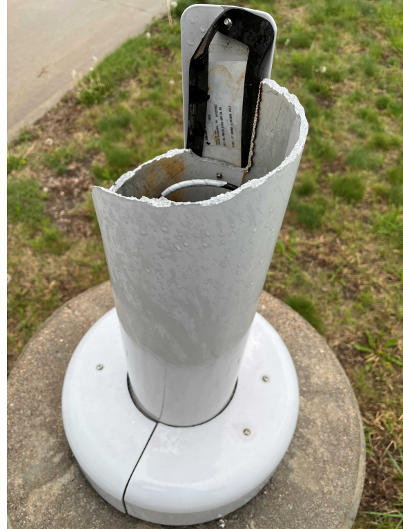
Failed light pole at handhole
