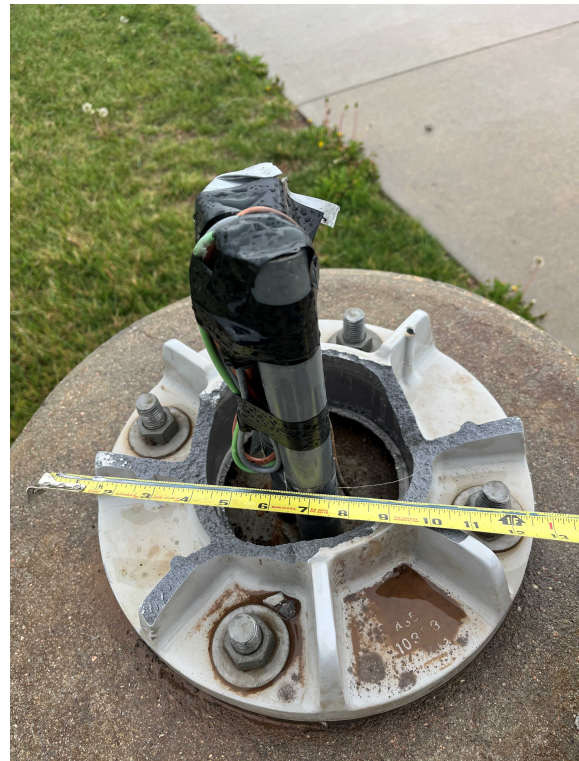
Failed light pole base casting
