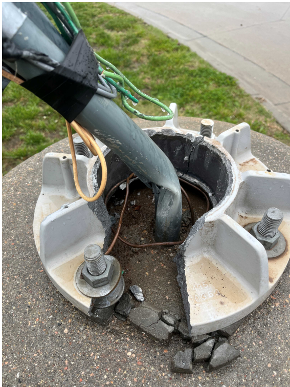
Failed light pole base casting
