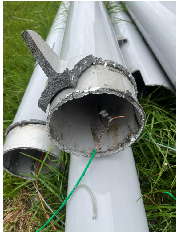
Failed light pole bases and base castings
