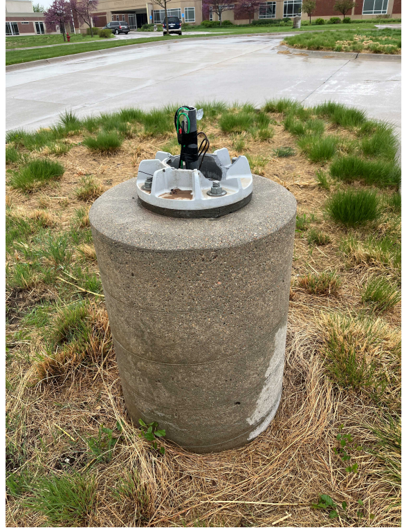
Failed light pole base casting
