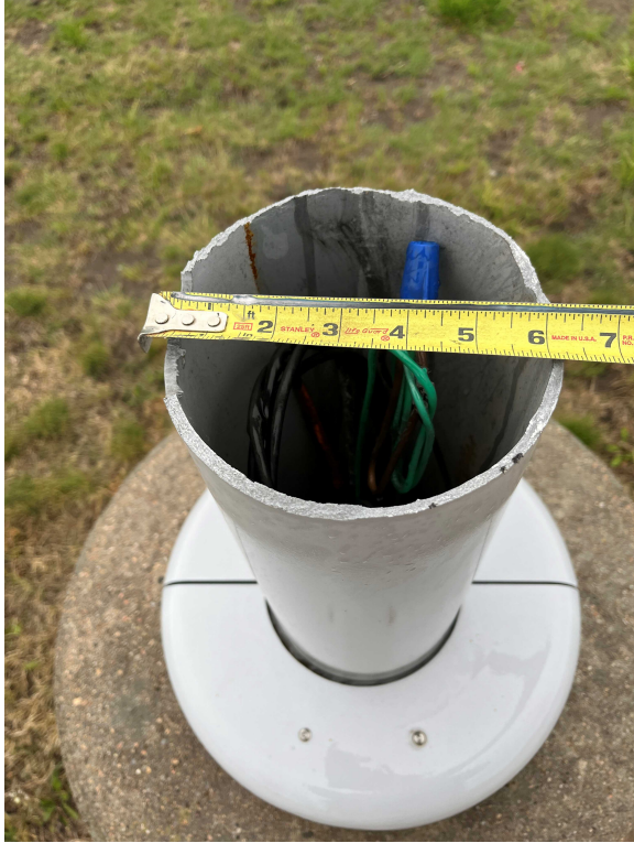
Failed light pole at handhole
