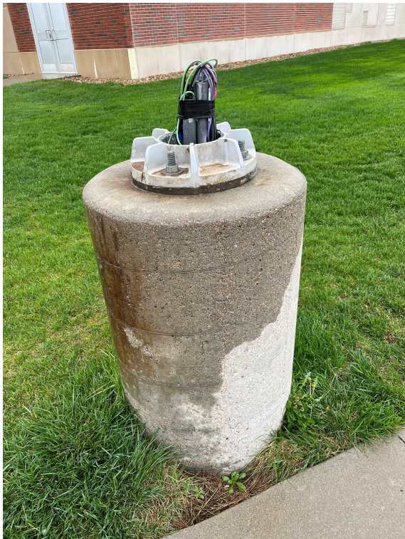
Failed light pole base casting
