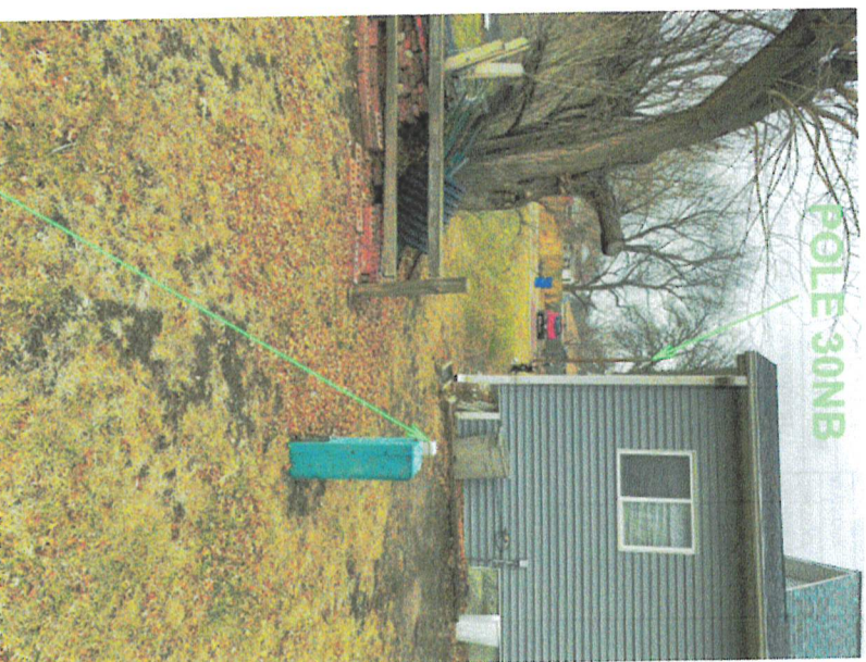
COPPER PED 35NB LOOKING NORTH
