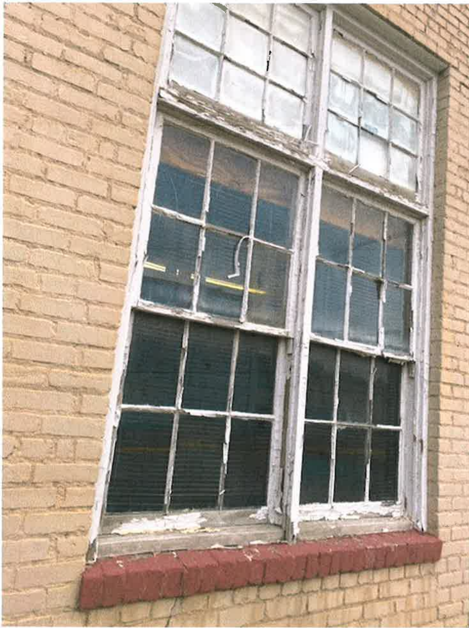
windows do not open and are rotten
