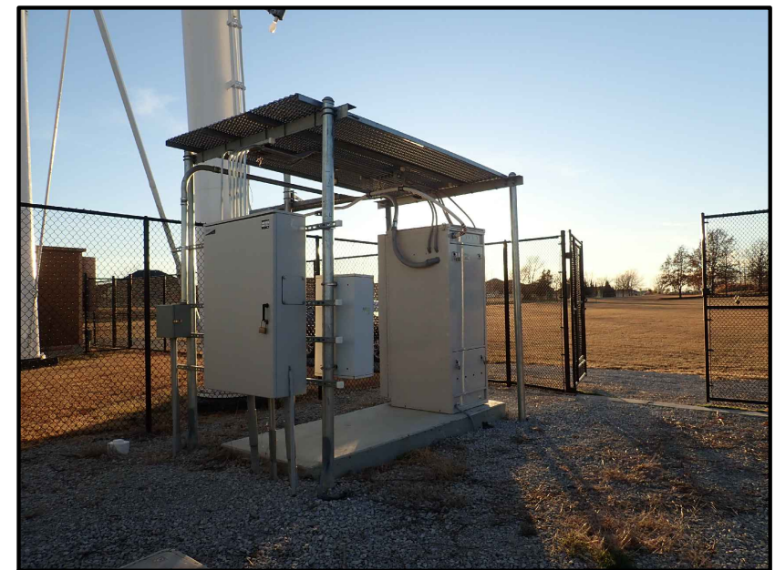
5 EQUIPMENT PAD PHOTO
