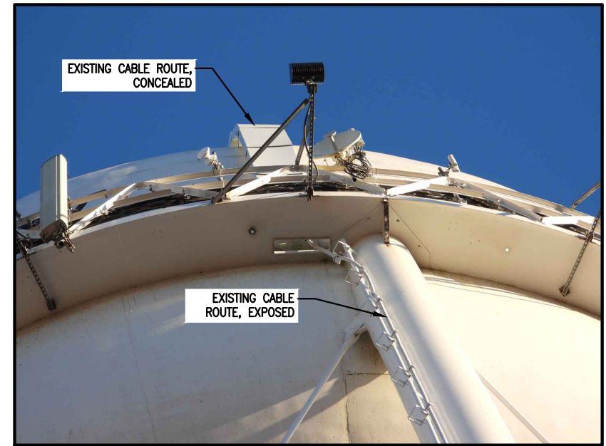
3 TOWER CABLE PHOTO
