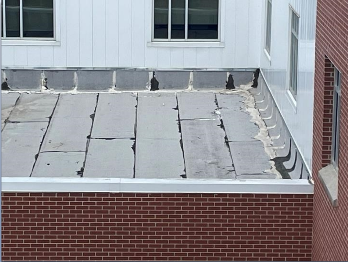
Image 1. Evidence of multiple leak repairs
