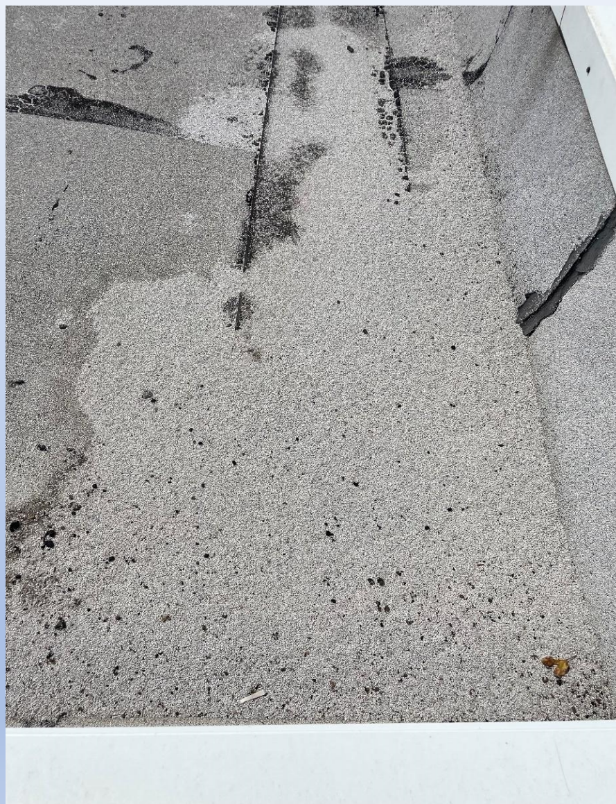
Image 4. Debris from asphalt deterioration collecting in corners of roof.
