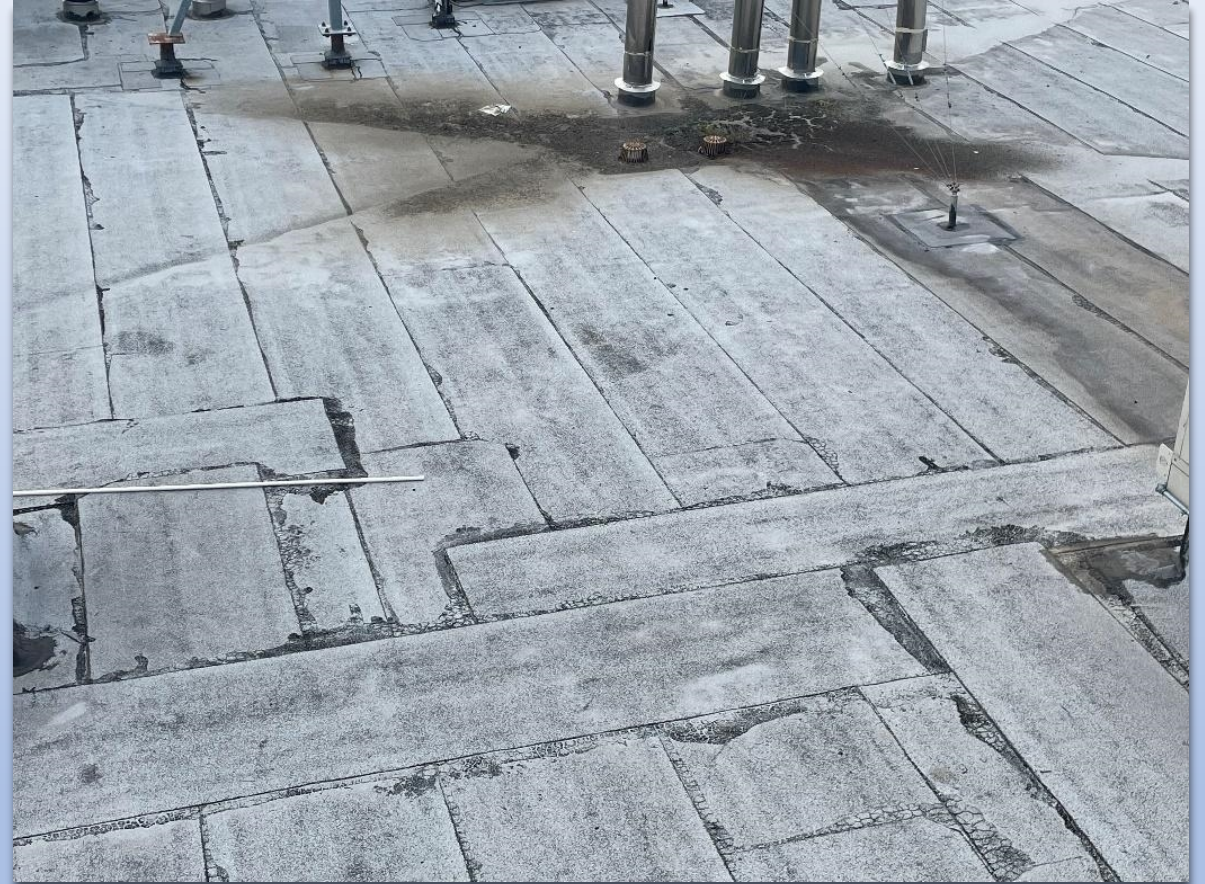
Image 2. Evidence of ponding water
