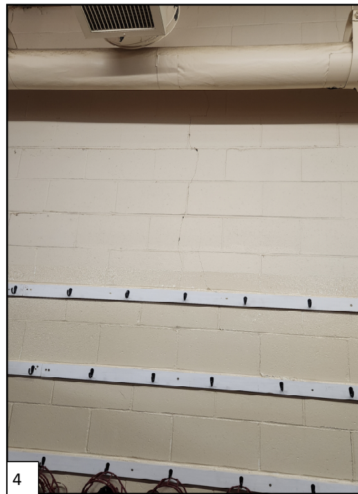
CMU Shrinkage Crack in Football Storage (non-structural)
