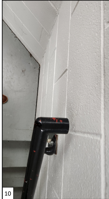
Separation of the wall from the Landing
