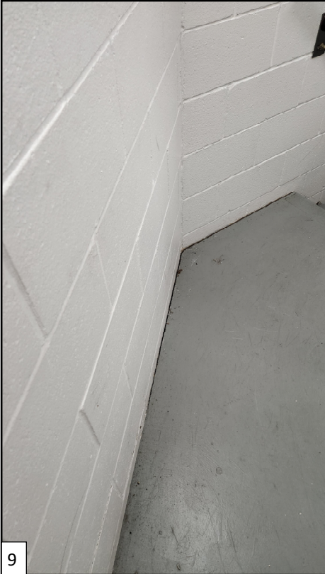
Separation of the wall from the Landing
