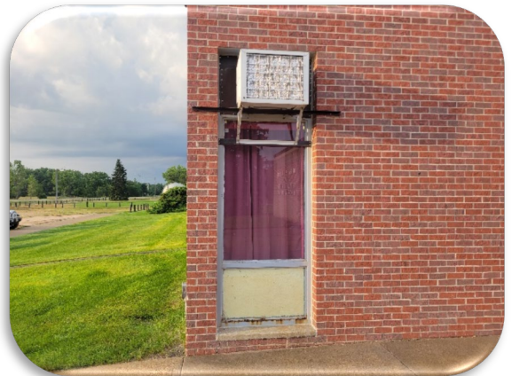
Exterior Windows – Some Frames Rusted Through
