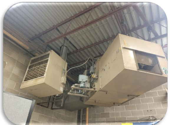
Shop Makeup Air Unit and Gas Unit Heater
