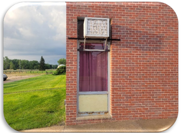
Exterior Windows – Some Frames Rusted Through
