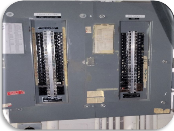
FPE Electrical Panels – Typical of Four
