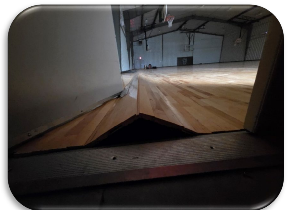
Activities Building Gym – Catastrophic Floor Damage
