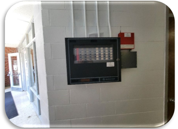
Update Antiquated Fire Alarm Control Panel & Devices
