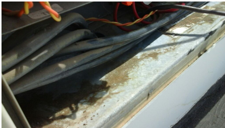
Photo showing visible water stains around holes that lead directly into the office. Repaired as part of the maintenance agreement.
