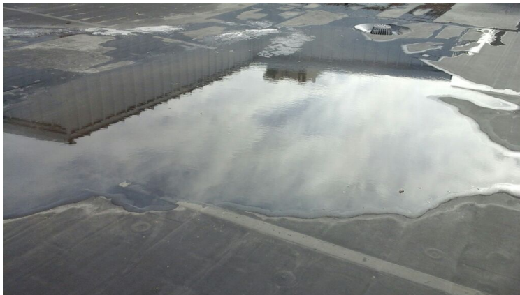
Photo showing ponding water near the drain.
