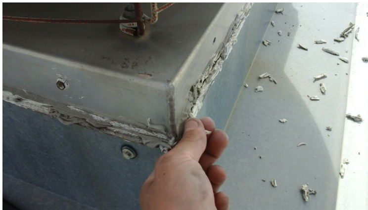
Photo showing projection with undersized metal flashing that was patched with multiple layers of caulking. Repaired as part of the maintenance agreement.
