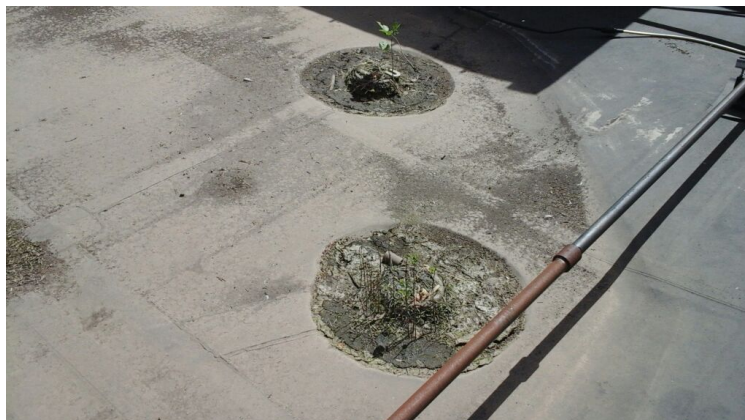
Photo showing drains clogged with debris over where a leak has been occurring. Cleaned out as part of the maintenance agreement.
