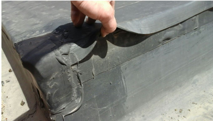
Photo showing a F patch over a former projection pulling up. Repaired as part of the maintenance agreement.
