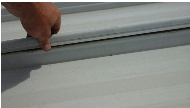
Photo showing a metal panel that is loose and open to weather.
