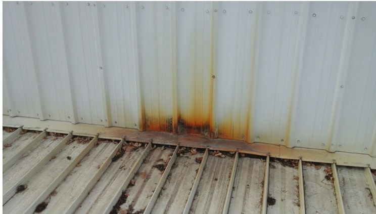
Photo showing area where the metal has started to rust.
