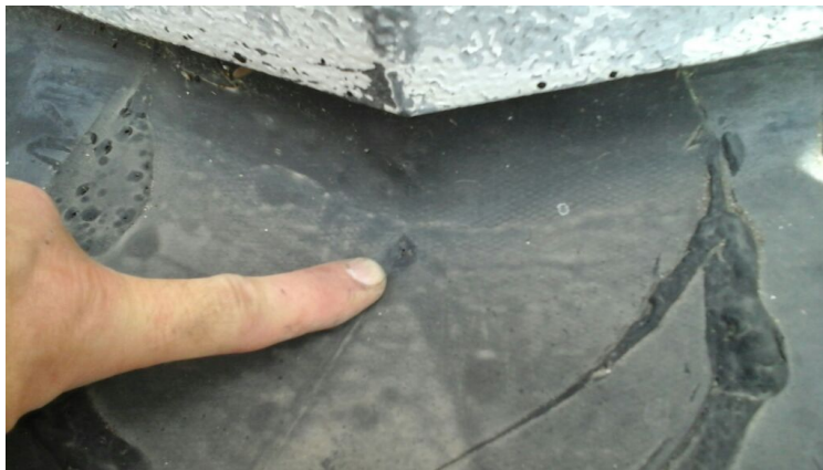
Photo showing a hole in a corner patch on the perimeter flashing. Repaired as part of the maintenance agreement.
