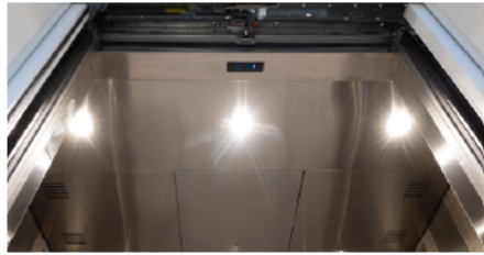
LED downlight ceiling
