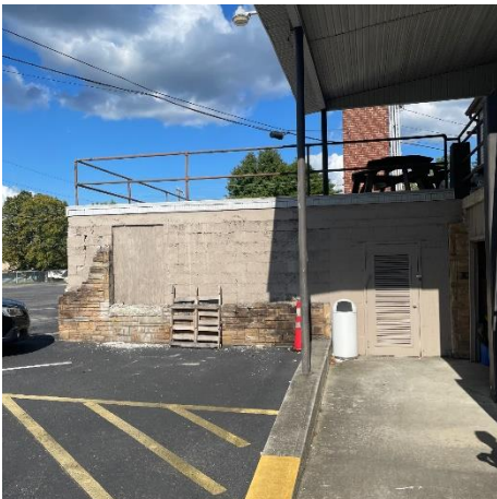
Photo #51 Back furnace room.
