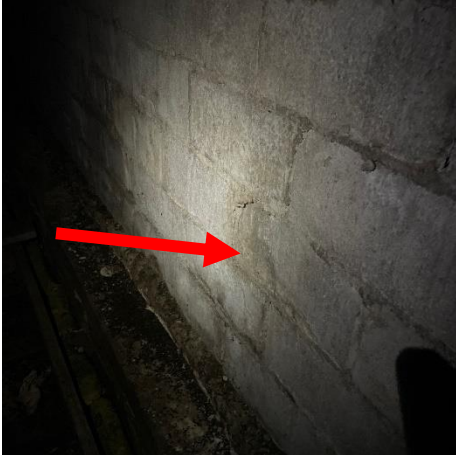
Photo #49 Mold Sample #5 location.
