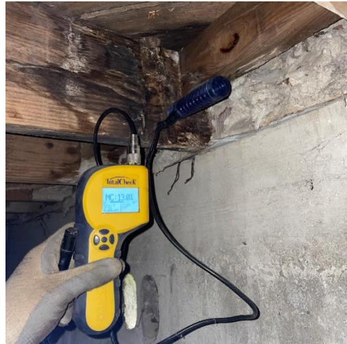
Photo #32 Moisture probed at near mold sample 2.
