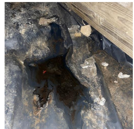
Photo #12 Typical standing water in crawlspace.
