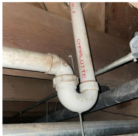
Photo #11 Moisture drops from plumbing in crawlspace.
