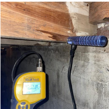
Photo #29 Moisture probing of possible moisture staining at joists at northwest elevation.
