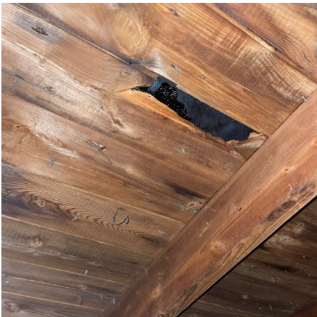
Photo #39 Isolated area of missing planking and roof system above without support.
