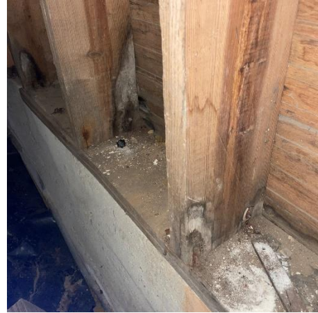
Photo #14 Wood deterioration observed at crawlspace vertical stud framing near Sample #1.
