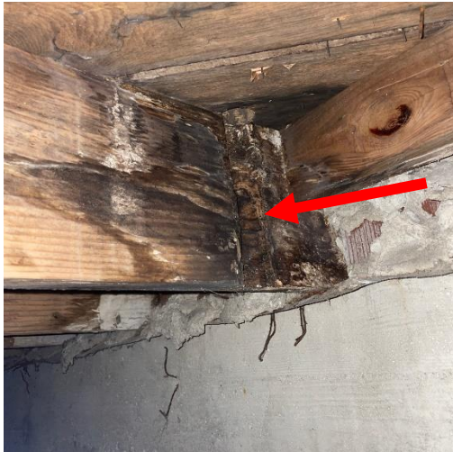
Photo #31 Joist framing at previous vertical plumbing line. Joist has been notched.
