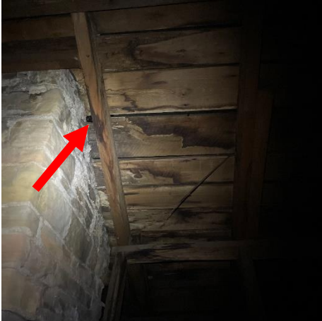
Photo #43 Location of deteriorated roof sheathing adjacent to the chimney.
