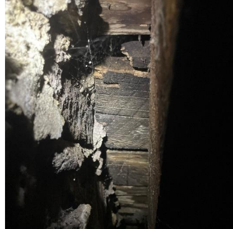
Photo #44 Sloped roof sheathing at chimney appeared to be deteriorated.
