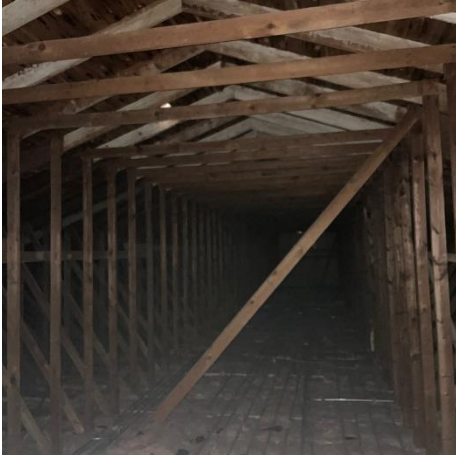
Photo #37 Fallen piece of bracing in attic.
