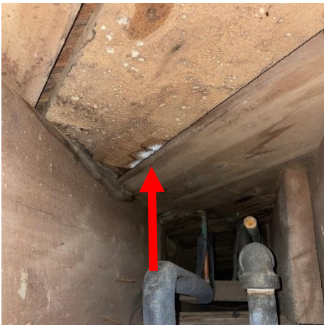
Photo #45 Mold Sample #1 location.
