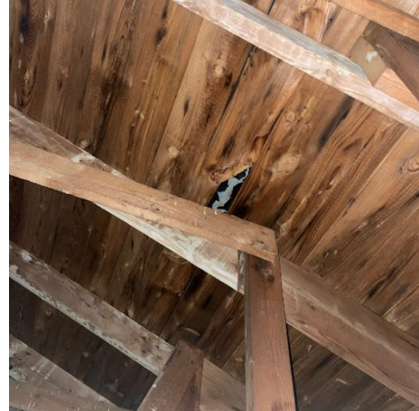
Photo #38 Isolated area of discontinuous roof plank decking and roof system above without support.
