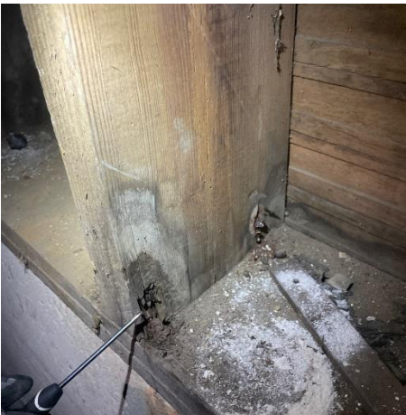
Photo #15 Wood deterioration observed at crawlspace vertical stud framing near Sample #1.
