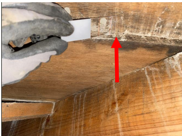
Photo #47 Mold sample #3 location. Typical tape lift sample in progress.
