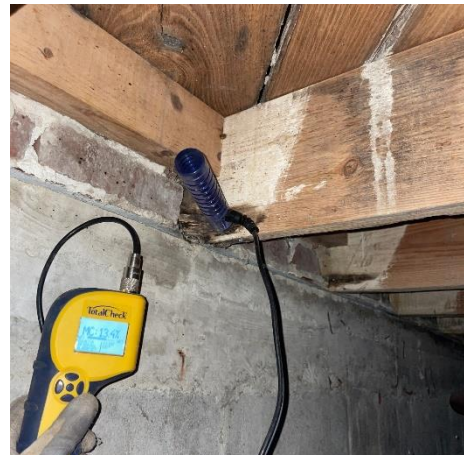
Photo #28 Moisture probe of joist at perimeter foundation connection.
