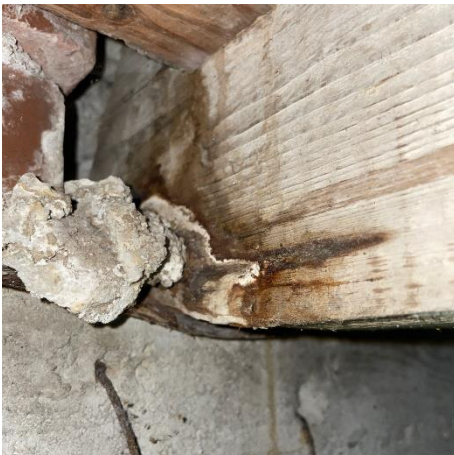
Photo #27 Close-up of joist connection at perimeter foundation at northwest elevation, near sample #2.
