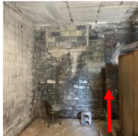
Photo #52 Typical furnace room condition and mold sample #7 location.
