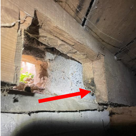
Photo #25 Rim joist cut at vent. Some wood deterioration observed in exterior moist joist at southeast elevation.
