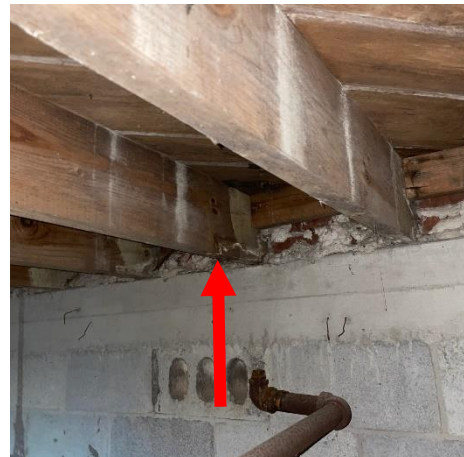
Photo #46 Mold Sample #2 location.
