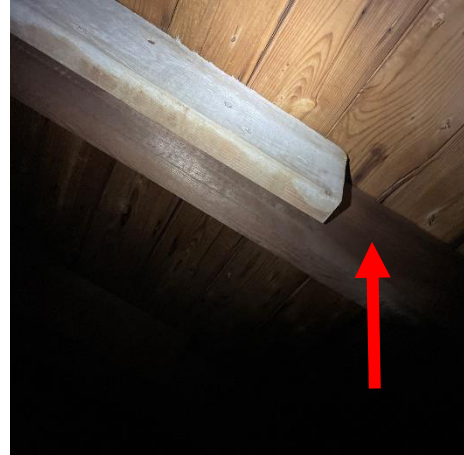
Photo #50 Mold sample #6 location.
