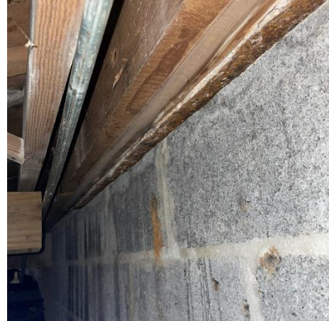
Photo #20 Rim joist condition near front building entrance. Moisture staining and deterioration noted.
