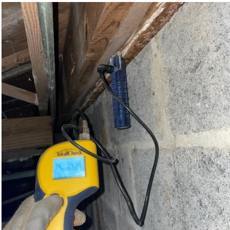
Photo #21 Elevated moisture content measurements at rim joist near building entrance.
