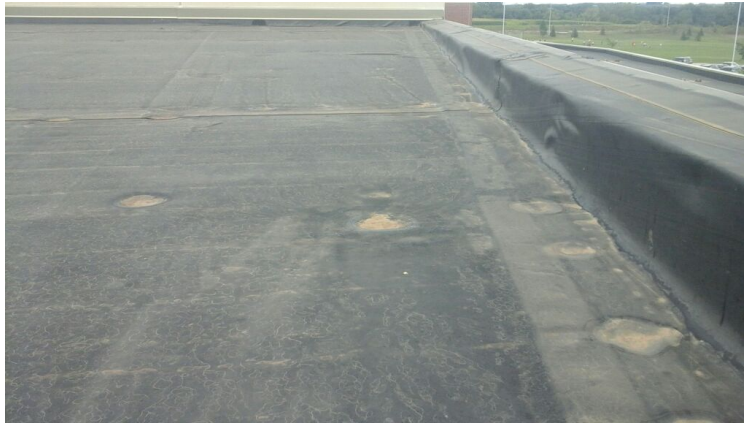
Photo showing condition of the perimeter flashings.
