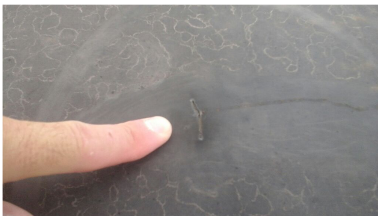
Photo showing a hole in the field membrane.
