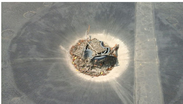
Photo showing clogged drain.
