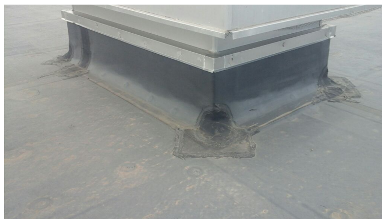
Photo showing condition of projection flashings.
