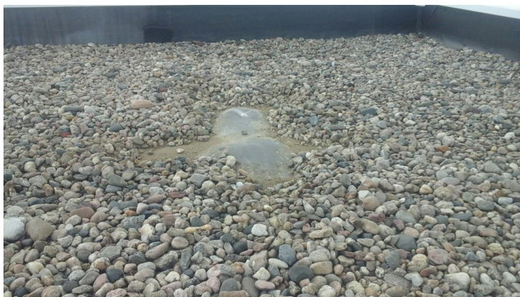
Photo showing additional area where isolation is extruding against the field membrane.
