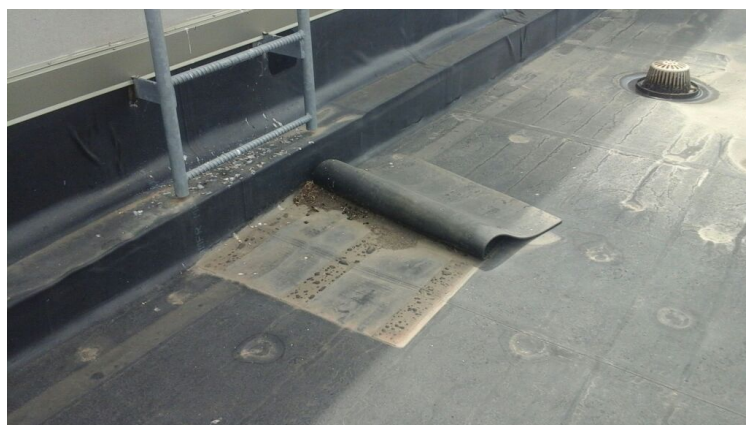
Photo showing walk pad under ladder pulling loose.
