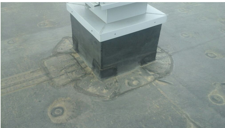
Photo showing condition of projection flashings.
