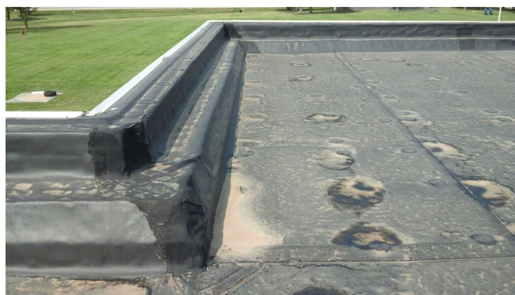
Photo showing condition of the perimeter flashings.
