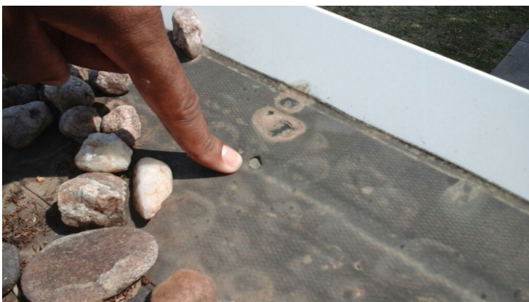
Photo showing an additional hole in the form flashings.
