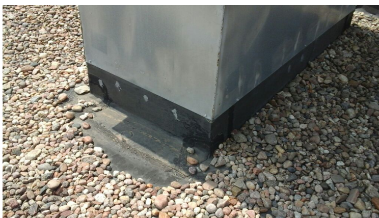
Photo showing condition of projection flashings.
