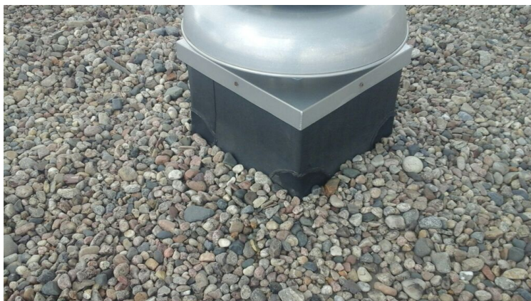
Photo showing condition of projection flashings.
