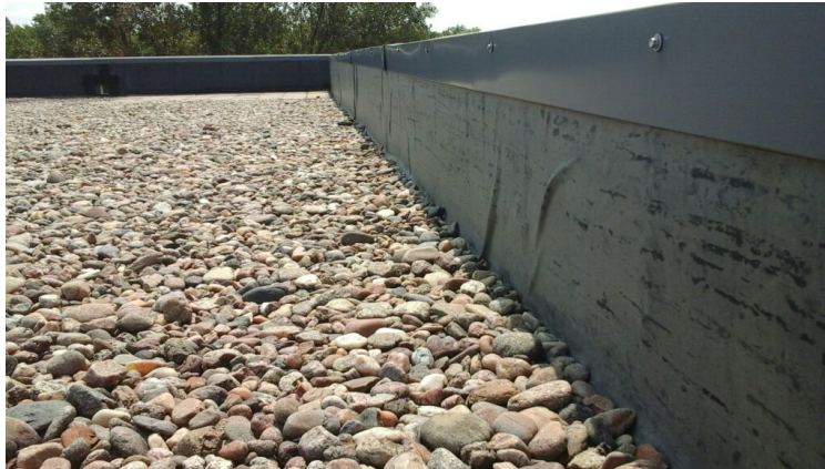
Photo showing condition of the perimeter flashings.
