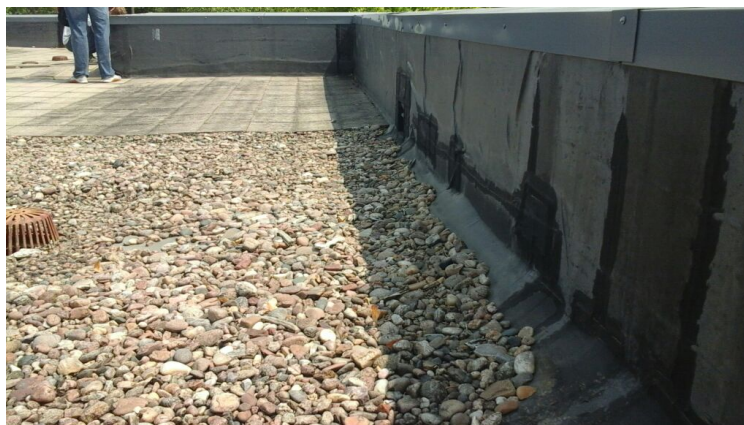
Photo showing condition of the perimeter flashings.
