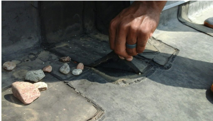
Photo showing a blowout patch in the perimeter flashing beginning to pull loose.
