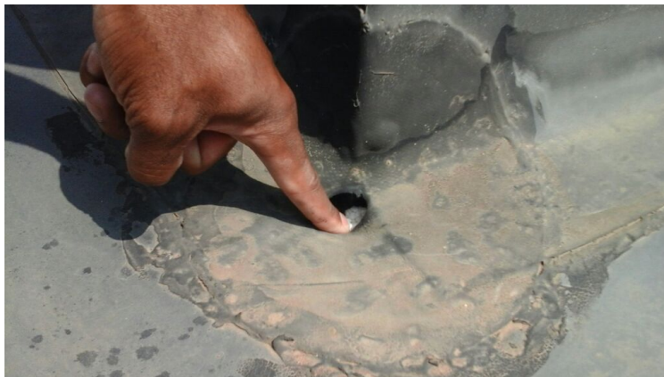
Photo showing a hole in the projection flashing where EPS is exposed.
