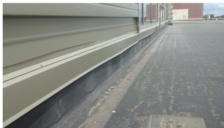
Photo showing condition of counter flashing under windows.
