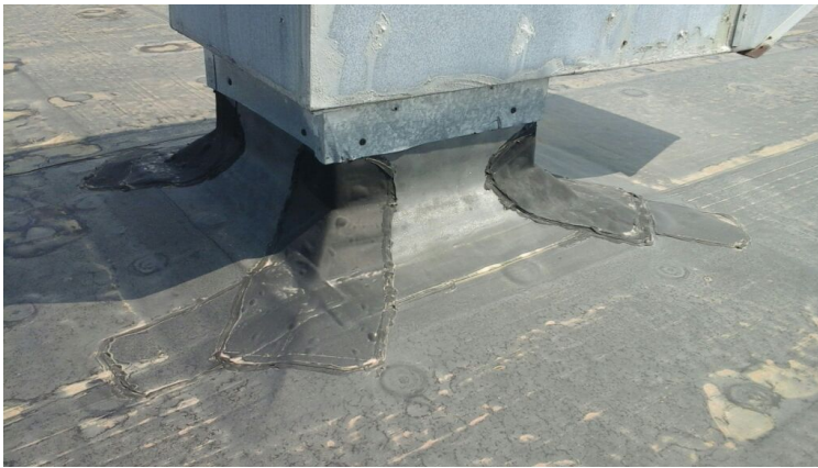
Photo showing condition of the projection flashings.
