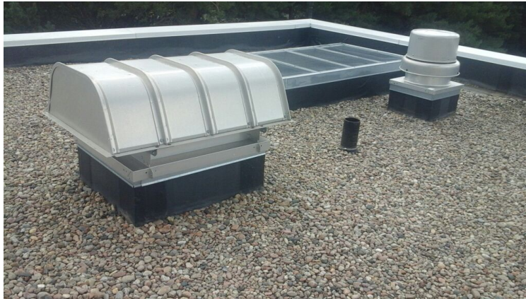
Photo showing condition of projection flashings.
