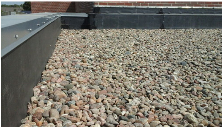
Photo showing condition of the perimeter flashings.
