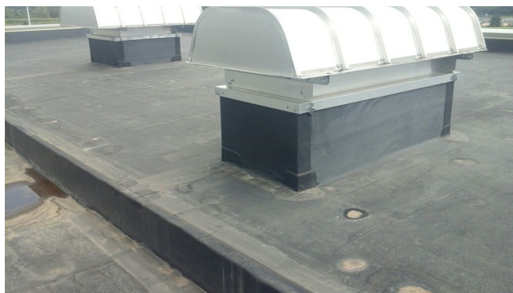
Photo showing condition of projection flashings.
