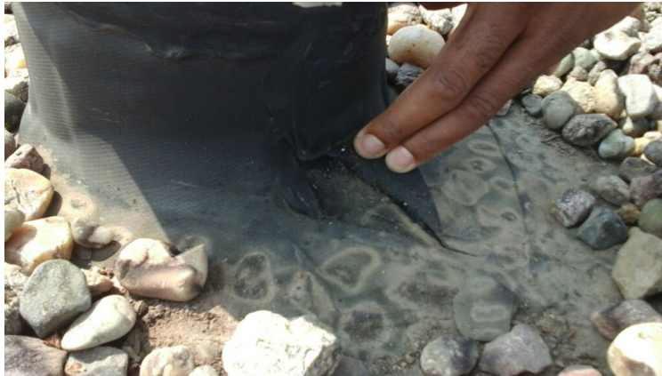
Photo showing flashing around projection that is pulling loose.
