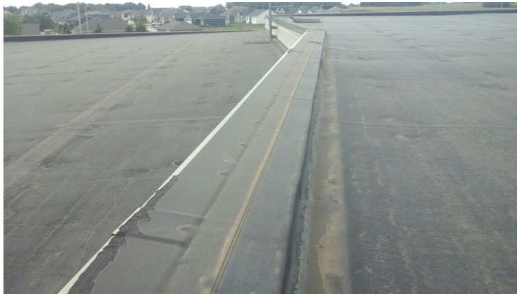
Photo showing condition of the form flashings.
