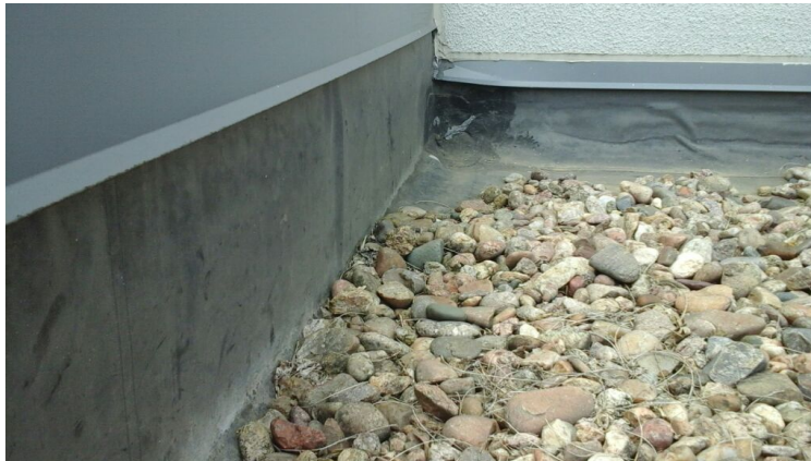
Photo showing condition of the perimeter flashings.
