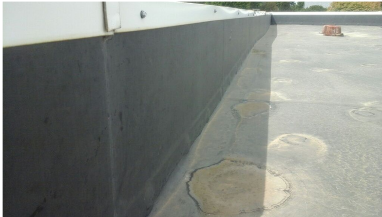
Photo showing condition of the perimeter flashings.
