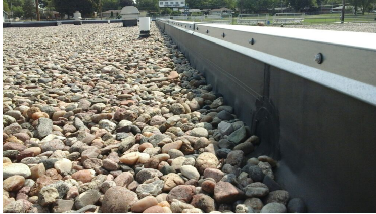
Photo showing condition of the perimeter flashings.
