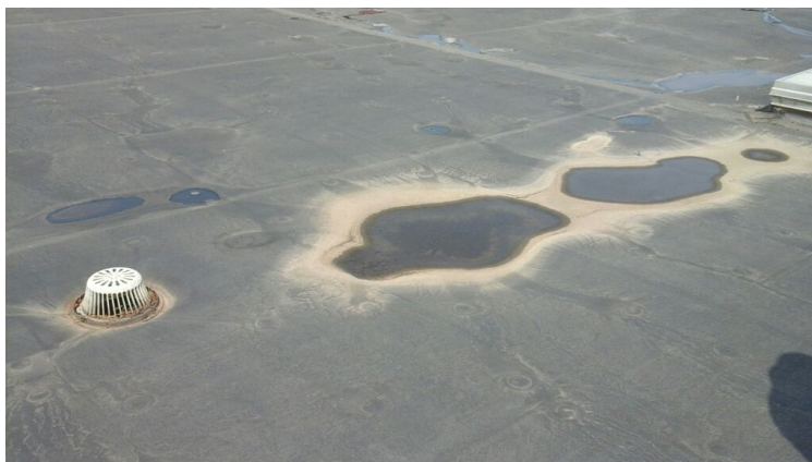
Photo showing minor ponding in the drain valley.
