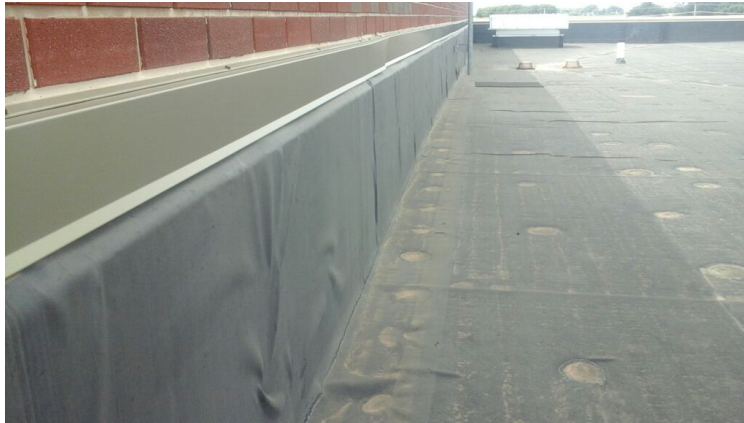
Photo showing condition of the perimeter flashings along brick wall.
