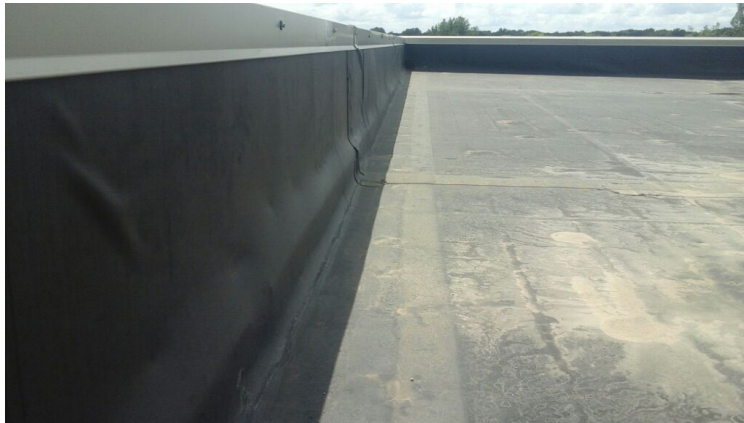
Photo showing condition of the perimeter flashings.
