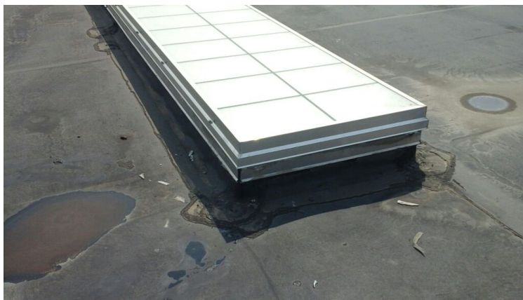
Photo showing condition of the skylight. Underside of counter flashing is caulked and likely preventing water from escaping. I recommend removing the excess caulking.
