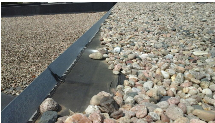
Photo showing condition of the form flashings.
