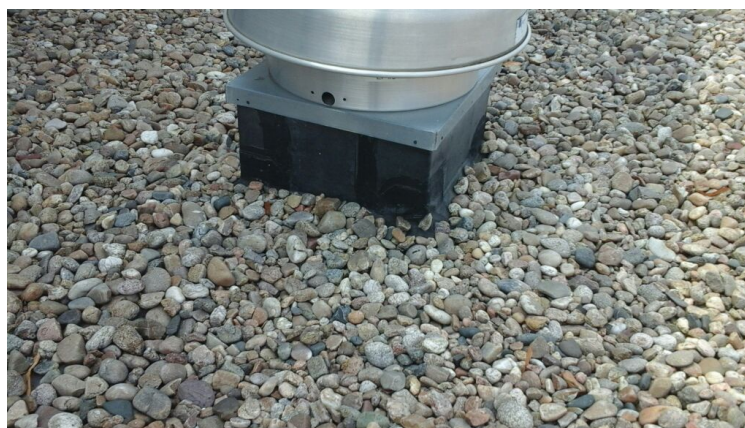
Photo showing condition of projection flashings.
