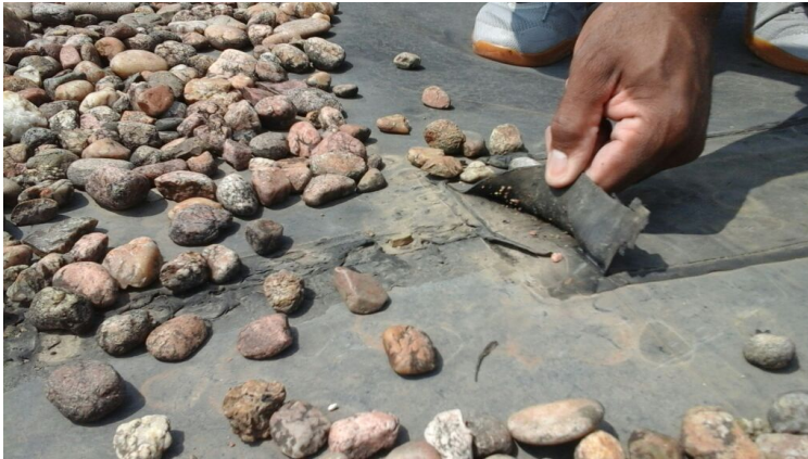
Photo showing patch pulling up along the seam.
