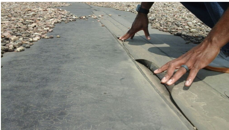
Photo showing patch along seam beginning to pull loose.
