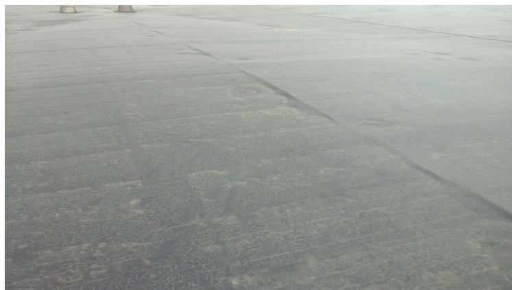
Photo showing minor cover board extrusion along cricket peak.
