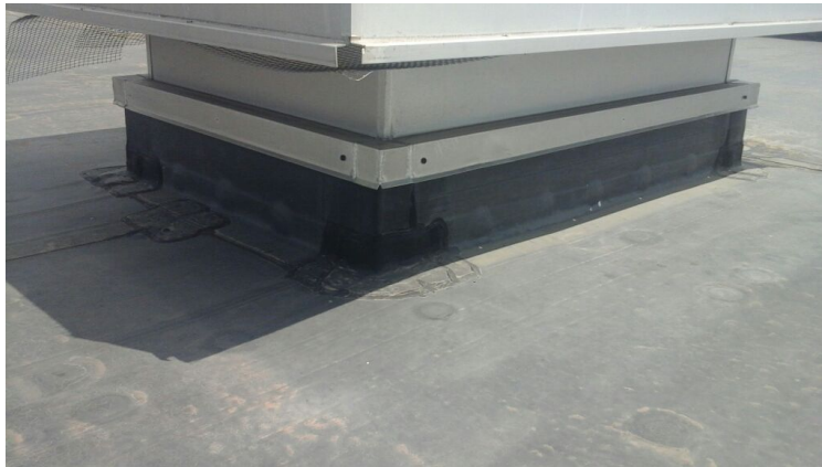
Photo showing condition of projection flashings.
