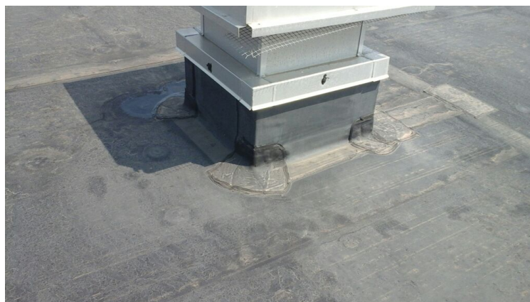
Photo showing condition of projection flashings.
