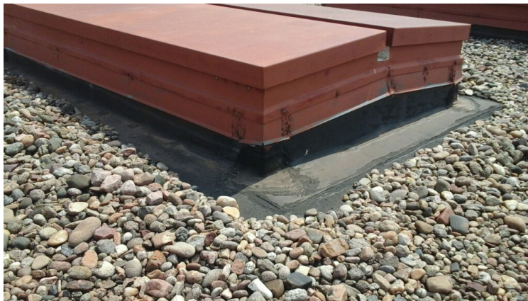
Photo showing condition of projection flashings.
