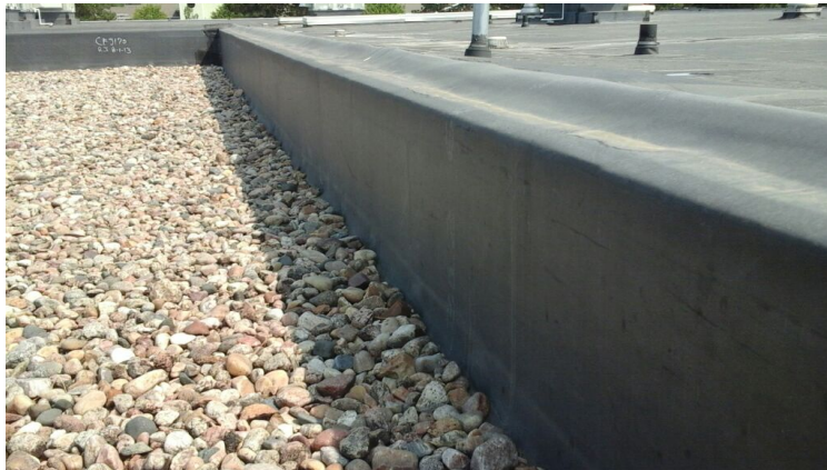
Photo showing condition of the perimeter flashings.
