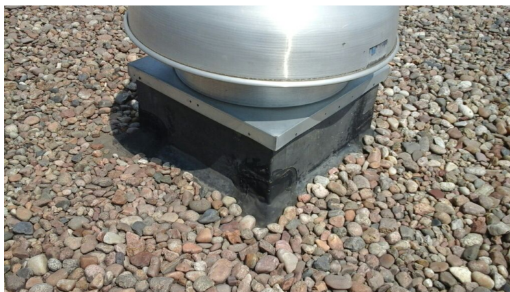
Photo showing condition of projection flashings.
