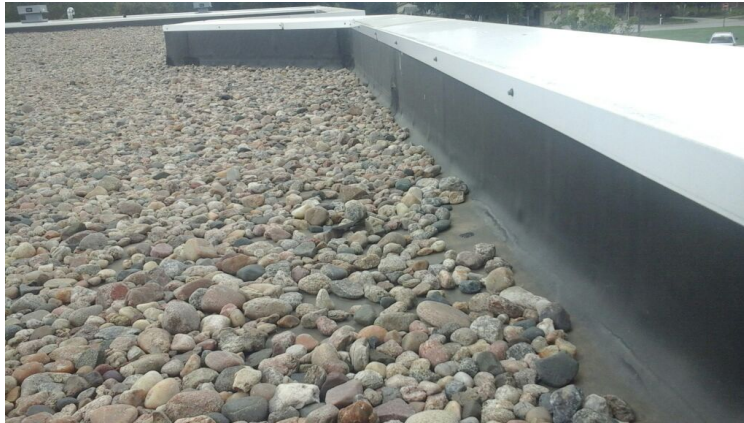
Photo showing condition of the perimeter flashings.
