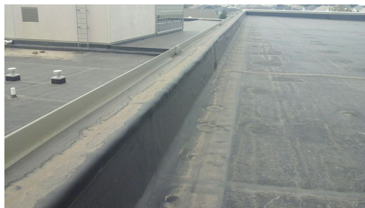
Photo showing condition of the form flashings.
