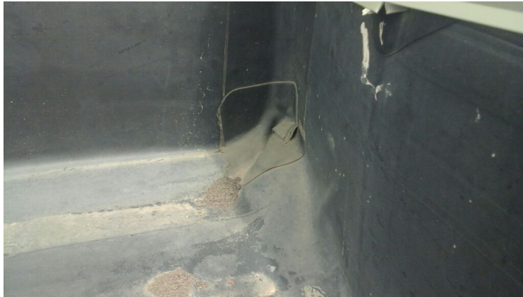
Photo showing minor tenting in the corner of the perimeter flashings.
