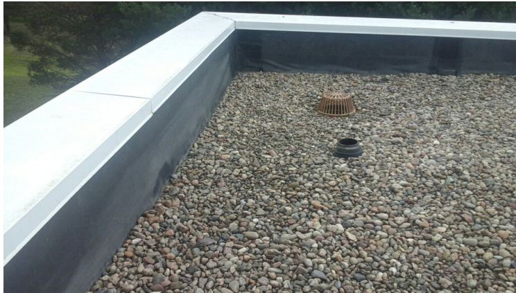
Photo showing tenting occurring corners.
