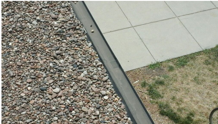
Photo showing condition of the form flashings.
