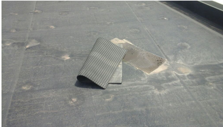
Photo showing loose walk pad.
