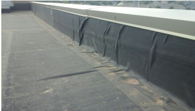
Photo showing some wrinkles in the perimeter flashing.
