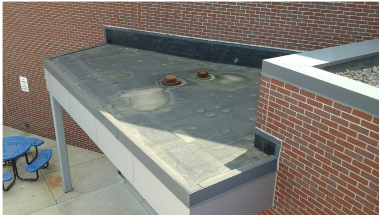
Photo showing overview of small Fully-adhered EPDM area adjacent to Area 11 Roof.
