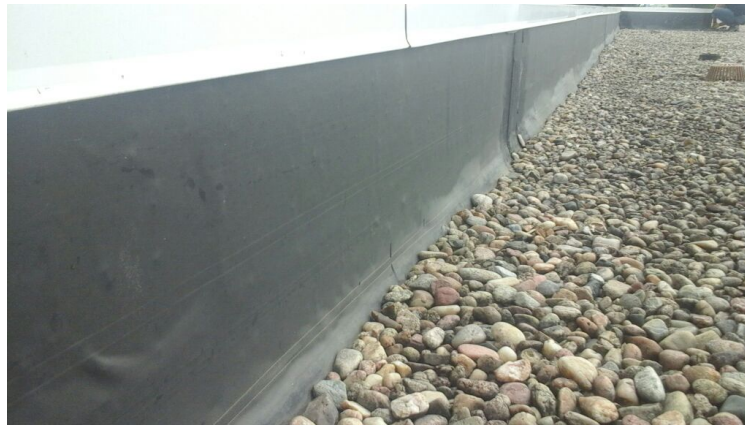
Photo showing additional tenting along the perimeter flashings.
