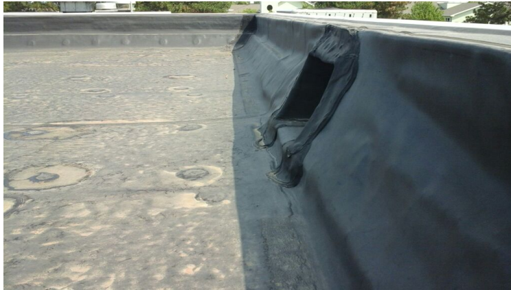
Photo showing condition of the perimeter flashings.
