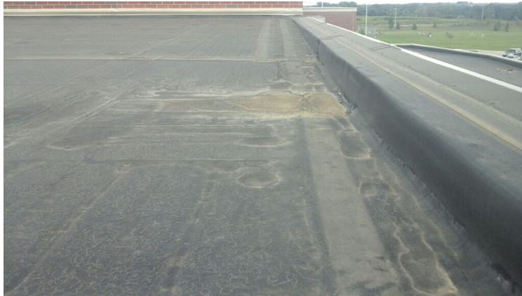
Photo showing condition of the perimeter flashings.
