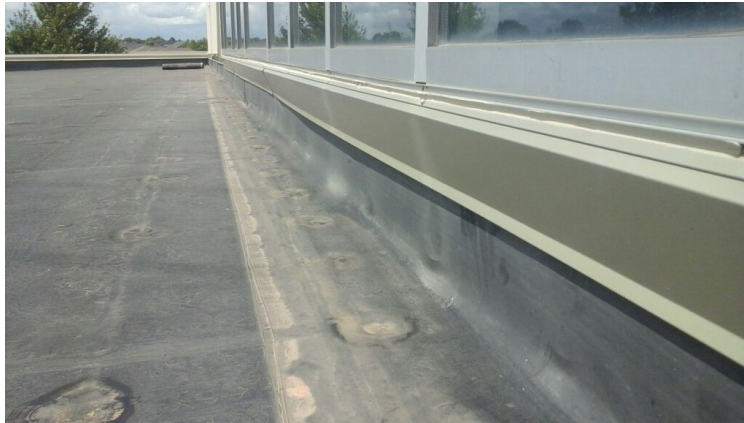
Photo showing condition of the counter flashing under the window wall.
