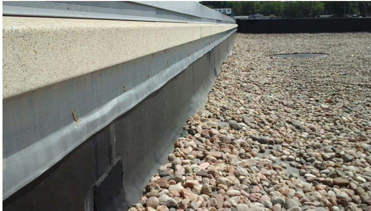
Photo showing condition of the perimeter flashings.
