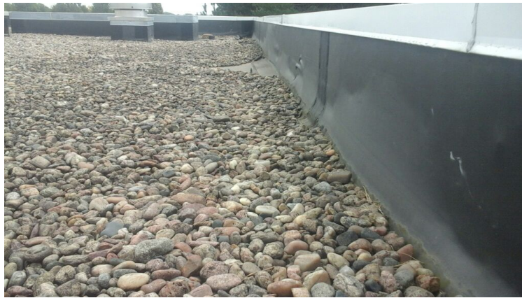
Photo showing tenting occurring along perimeter flashing and into corner.
