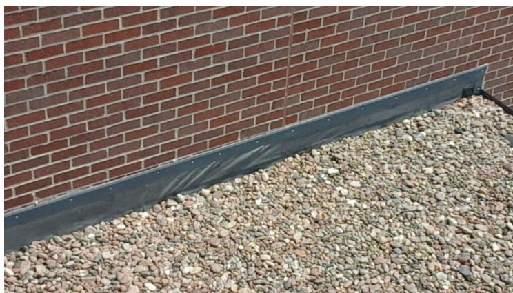
Photo showing condition of the perimeter flashings.
