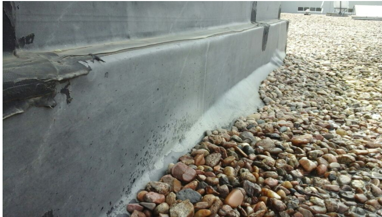
Photo showing tenting along the projection flashings.
