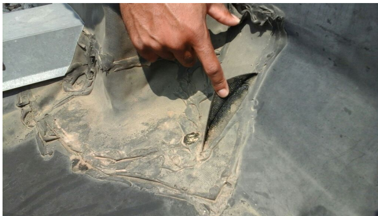
Photo showing additional blowout patch pulling loose.
