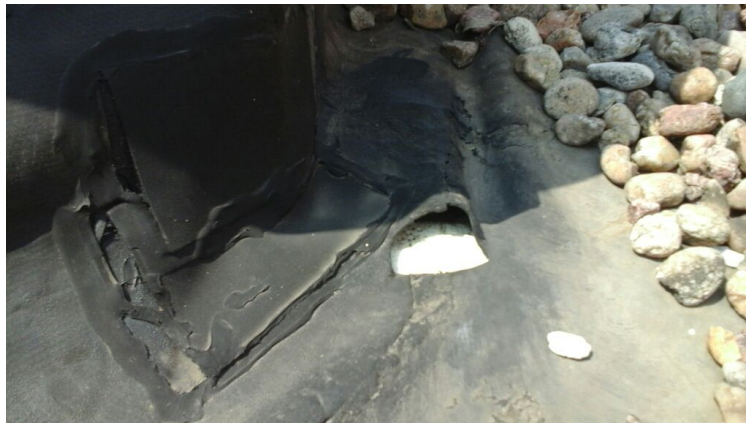
Photo showing a hole in the tenting projection flashings where EPS is exposed.
