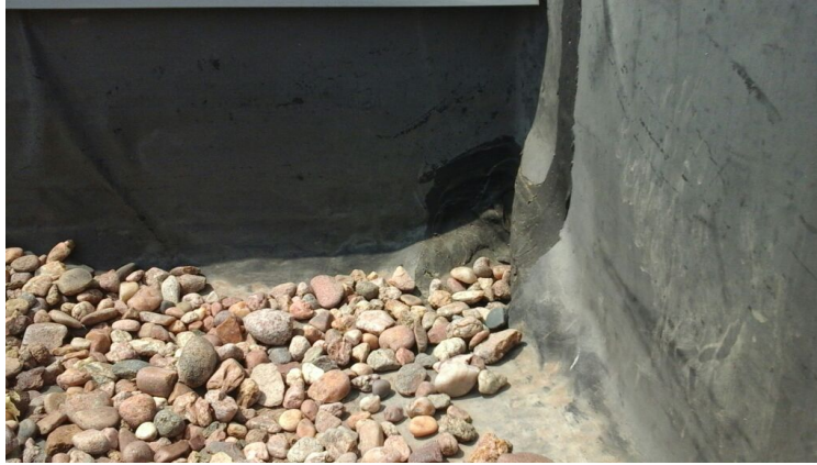
Photo showing tenting occurring in the corner of the perimeter flashings.
