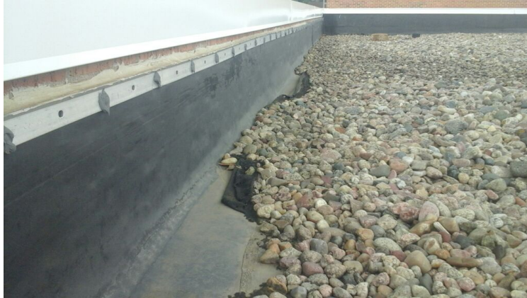
Photo showing where metal does not cover term bar.
