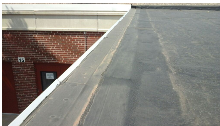
Photo showing condition of the form flashings.
