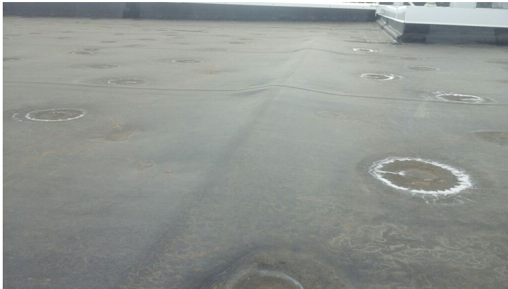
Photo showing coverboard extruding under field membrane due to joints not being staggered on install.
