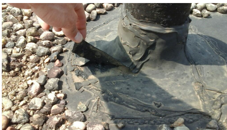
Photo showing flashing around soil stack beginning to pull loose.
