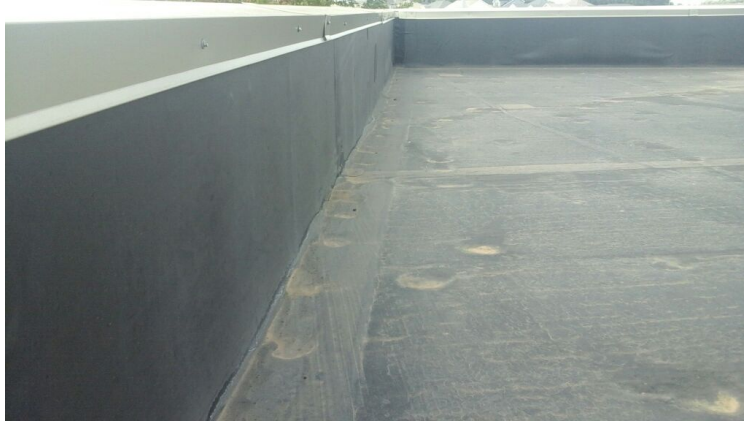
Photo showing condition of the perimeter flashings.
