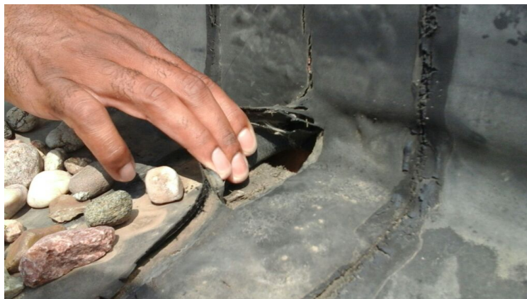
Photo showing a hole in the perimeter flashing. The decking is exposed and this is almost certainly a leak.
