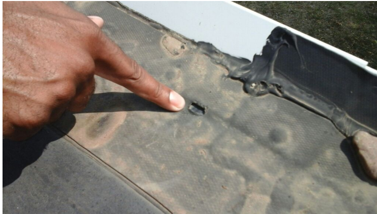
Photo showing a hole in the form flashings.
