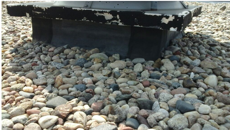
Photo showing condition of projection flashings.
