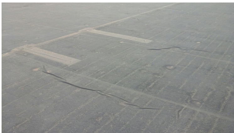
Photo showing minor wrinkles in the field membrane.
