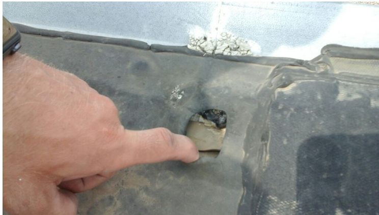
Photo showing a hole in the form flashings exposing interior.
