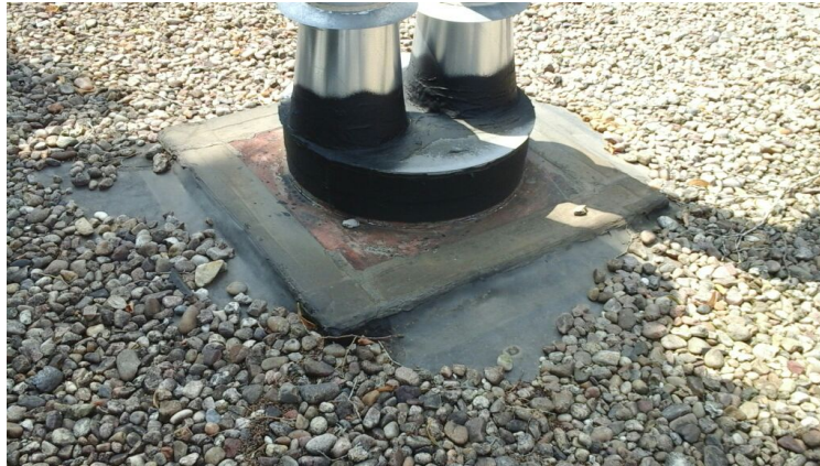
Photo showing condition of low projection flashings.
