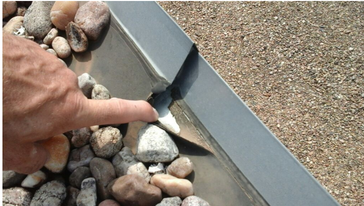
Photo showing form flashings opening up due to metal displacement.
