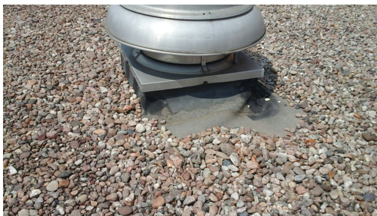
Photo showing tenting along the projection flashings.
