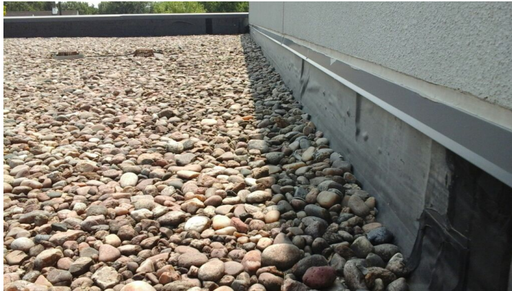
Photo showing condition of the perimeter flashings along the EIFS wall.
