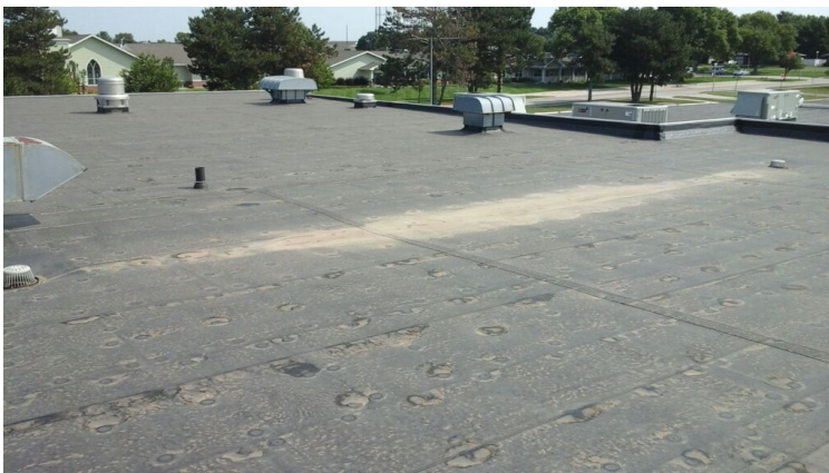
Photo showing evidence of ponding water in the drain valley.
