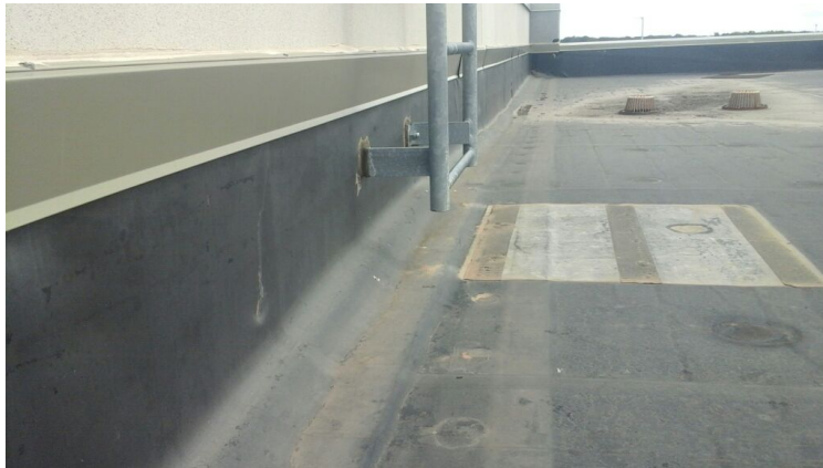
Photo showing condition of the perimeter flashings under ladder.
