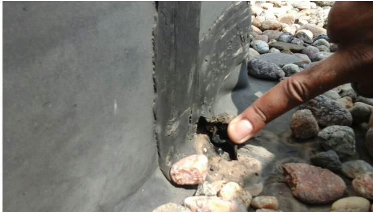
Photo showing projection flashings beginning to pull loose.
