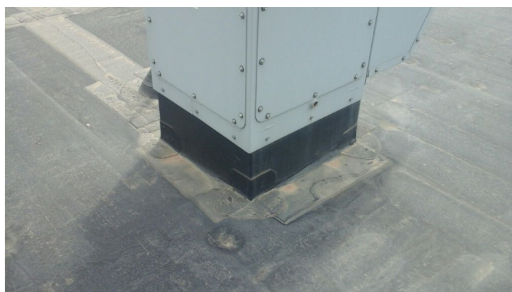
Photo showing condition of projection flashings.
