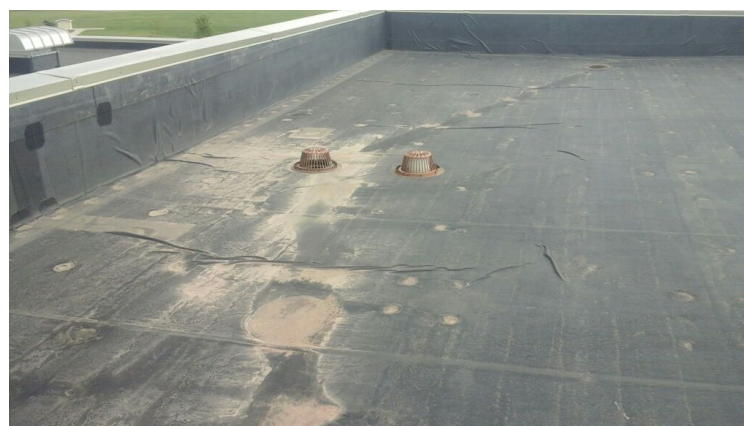
Photo showing minor wrinkles in the drain valley.
