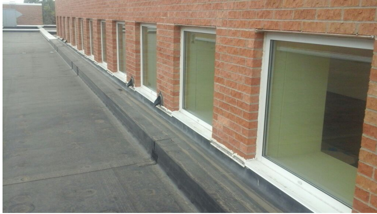
Photo showing condition of the perimeter flashings along window wall.
