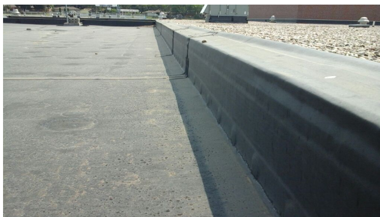
Photo showing condition of the perimeter flashings.
