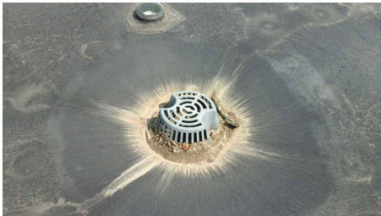
Photo showing additional clogged drain.
