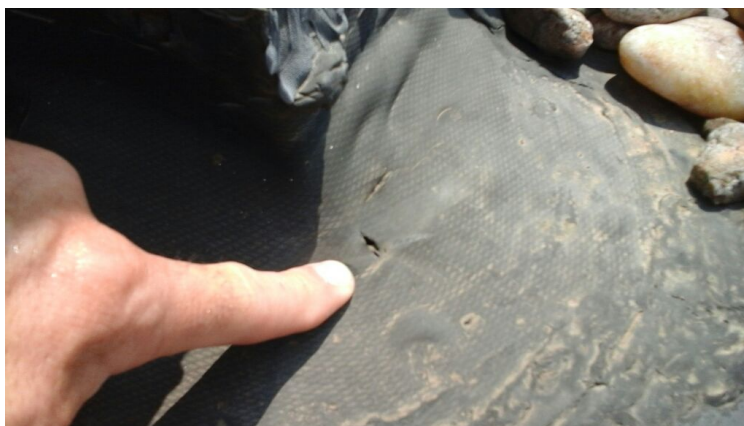
Photo showing a hole in the projection flashing.
