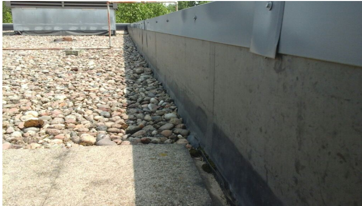
Photo showing condition of the perimeter flashings.
