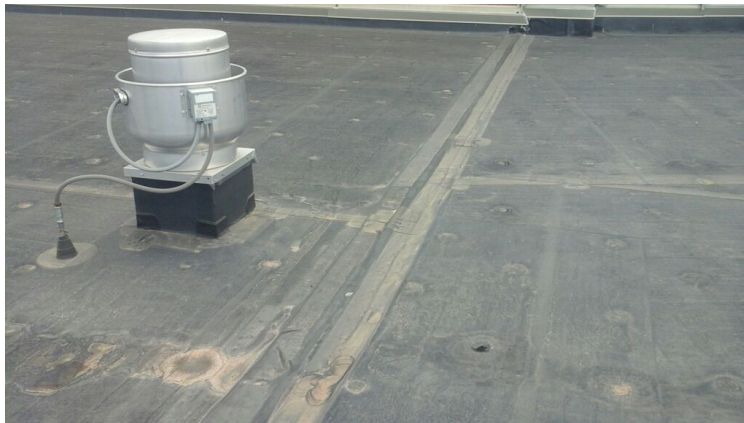
Photo showing condition of the expansion joint.
