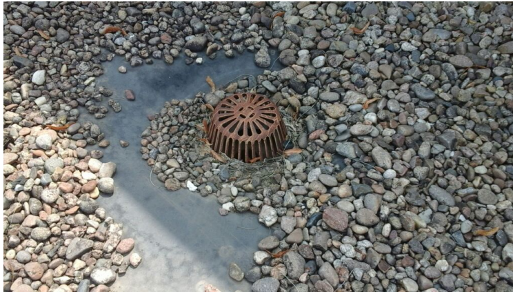
Photo showing clogged drain.
