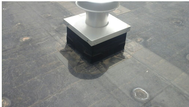
Photo showing condition of projection flashings.
