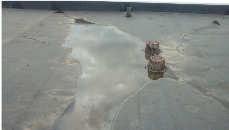
Photo showing ponding water due to lack of sump.
