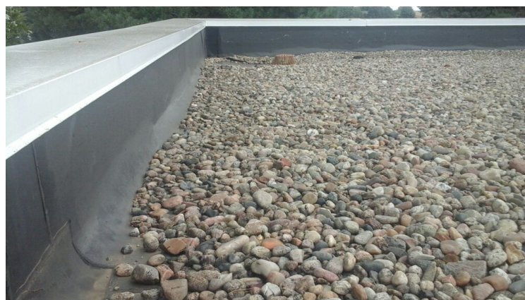
Photo showing minor tenting along the perimeter flashings.
