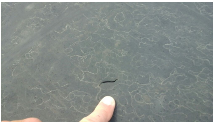
Photo showing a hole in the field membrane that is allowing water to penetrate interior.
