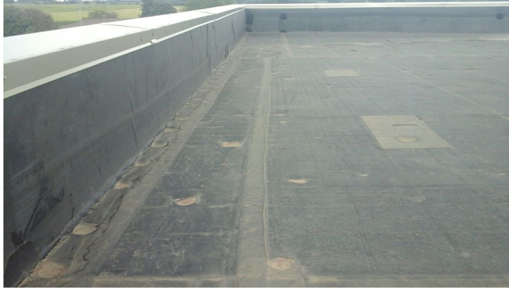
Photo showing condition of the perimeter flashings.
