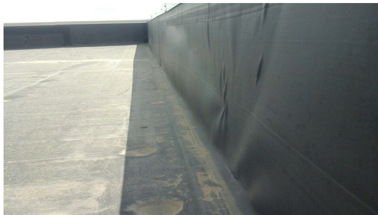
Photo showing minor delamination along the parapet wall.
