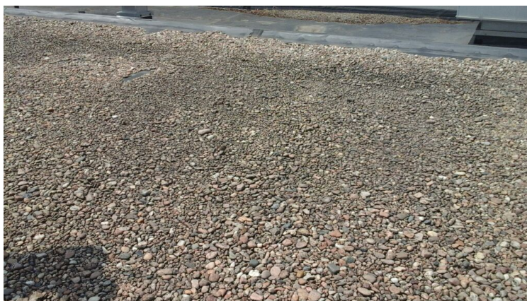
Photo showing evidence of ponding water.
