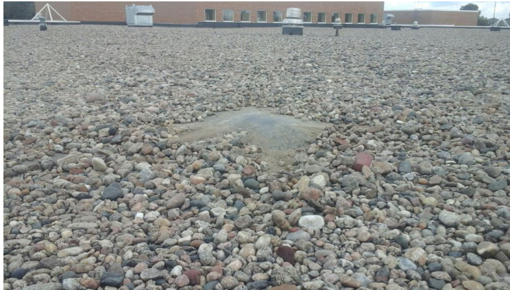
Photo showing area where insulation is pushing up on membrane.
