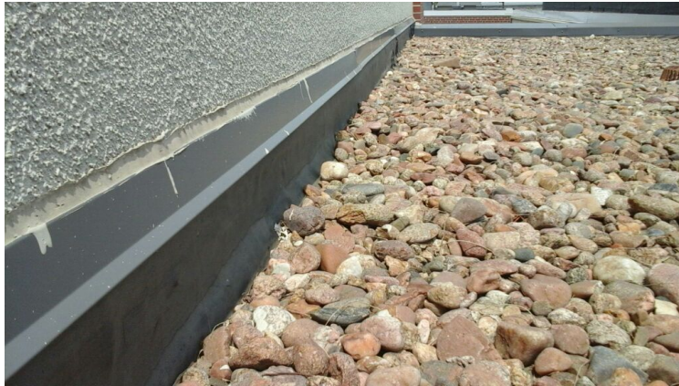
Photo showing condition of the perimeter flashings under the EIFS.
