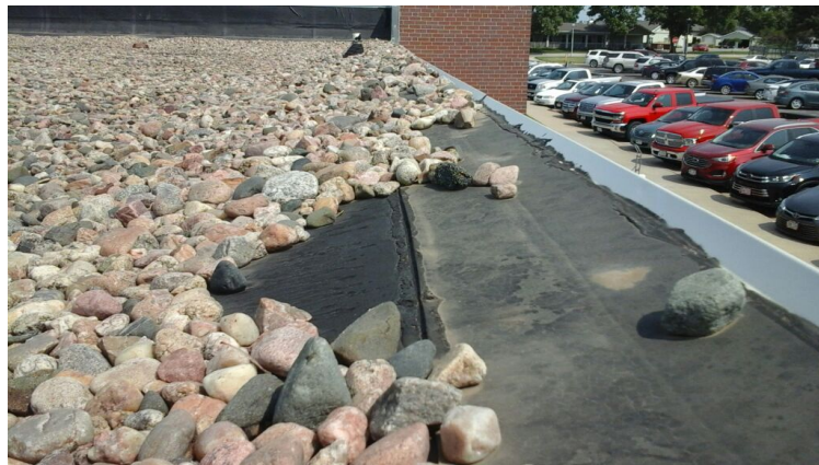
Photo showing condition of form flashing along perimeter edge.
