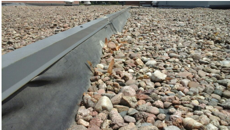
Photo showing minor tenting along the interior perimeter flashings.
