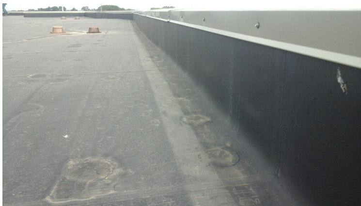
Photo showing condition of the perimeter flashings.
