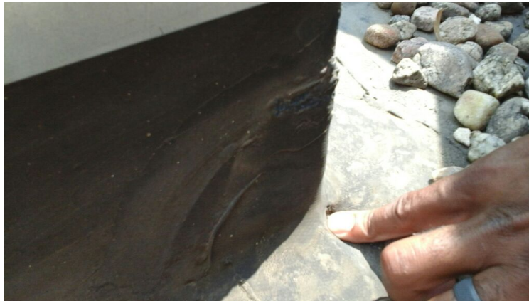
Photo showing another hole in a projection flashing.
