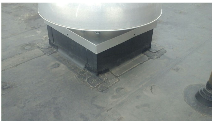
Photo showing condition of projection flashings.
