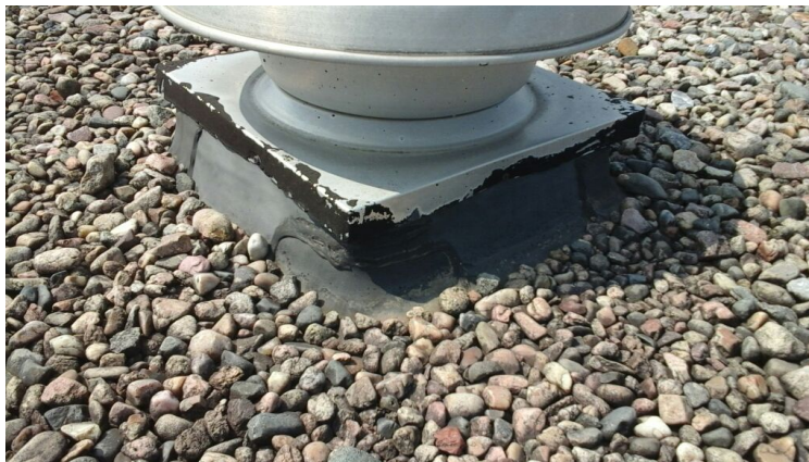
Photo showing condition of projection flashings.
