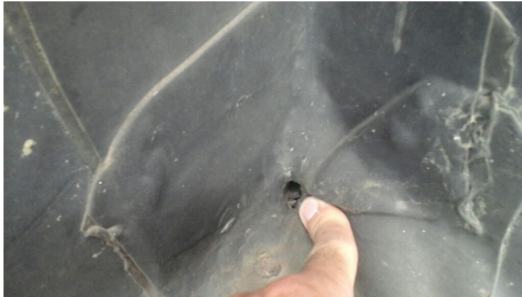
Photo showing a hole in the corner of the perimeter flashings.
