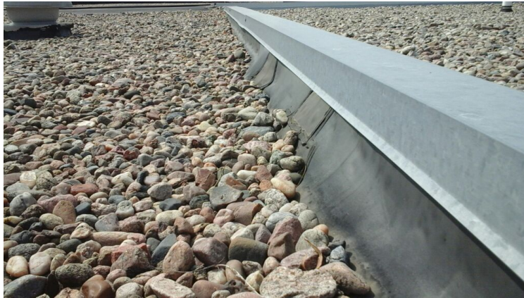
Photo showing tenting along the expansion joint.
