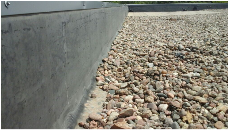
Photo showing condition of the perimeter flashings.
