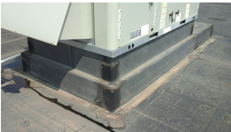
Photo showing condition of projection flashings.
