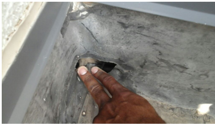
Photo showing patch in the perimeter flashing pulling loose.
