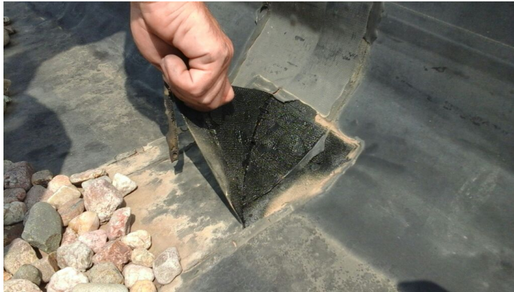
Photo showing a blowout patch on the perimeter flashing pulling loose.
