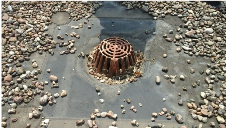
Photo showing a slightly clogged drain.
