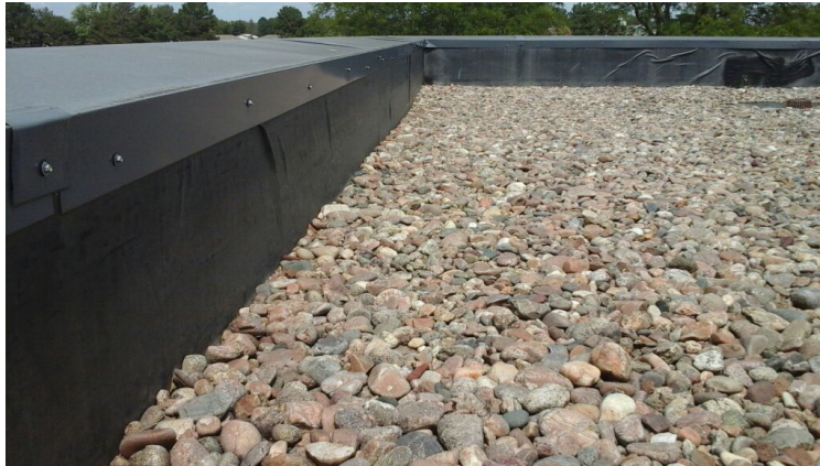
Photo showing condition of the perimeter flashings.
