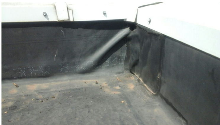
Photo showing condition of the perimeter flashings in the corner.
