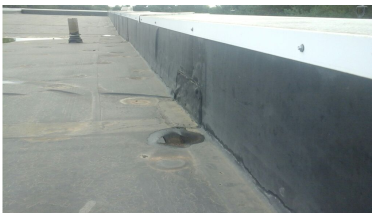
Photo showing condition of the perimeter flashings.
