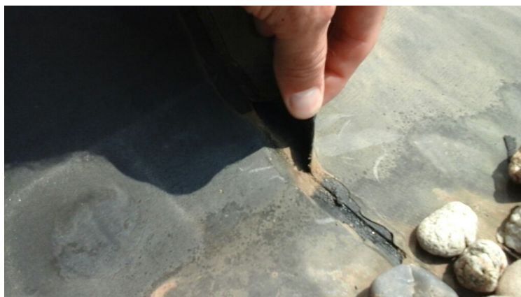
Photo showing additional blowout patch on perimeter pulling loose.
