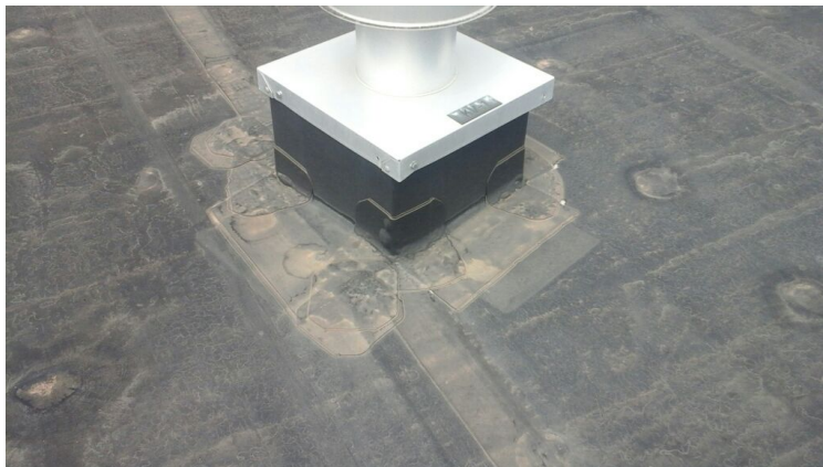
Photo showing condition of projection flashings.
