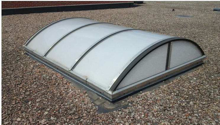
Photo showing condition of the skylight.
